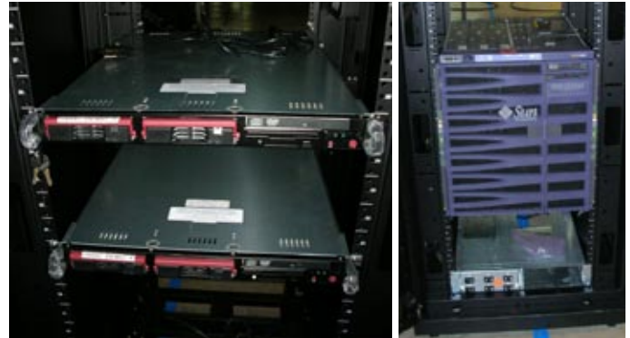
Figure 2. Servers modified to accept 380V DC
