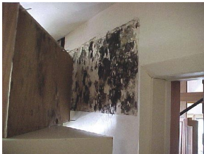
Figure 2. Some mold is hidden from view, such as the mold shown in this image, which was discovered when cabinets were removed from a wall (Photo courtesy of Mike McNickle)
