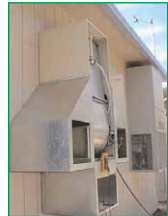
Figure 1. This HVAC system was designed for the relocatable classroom study.
