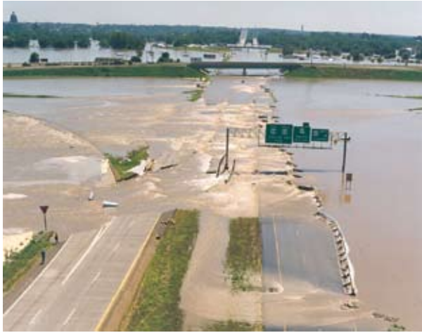
The Great Flood of 1993 caused flooding along 500 miles of the Mississippi and Missouri river systems. The photo shows its effects on U.S. Highway 54, just north of Jefferson City, Missouri.
