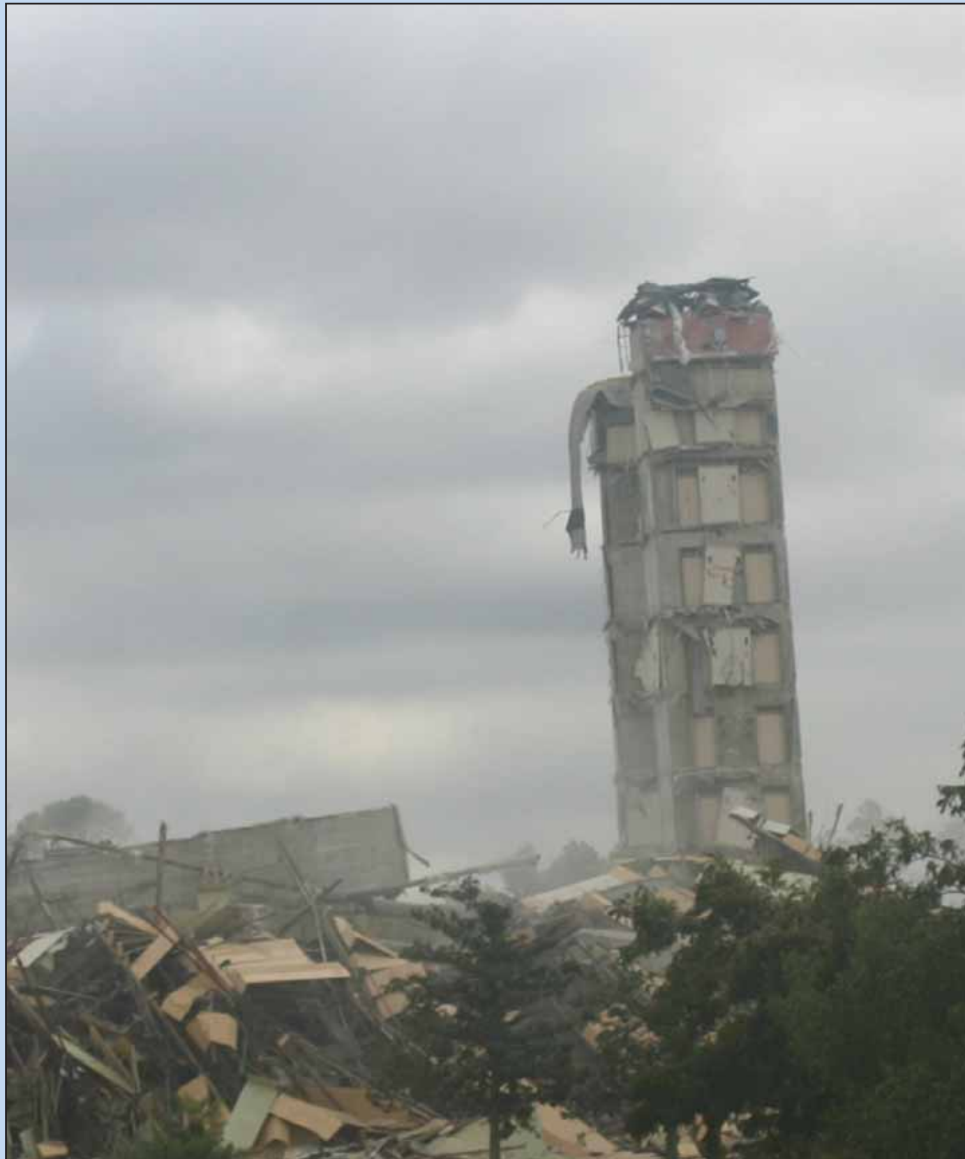
Two stubborn stairwells remained standing when all the dust settled. The demolition contractor will use a wrecking ball to push the structures completely down.
