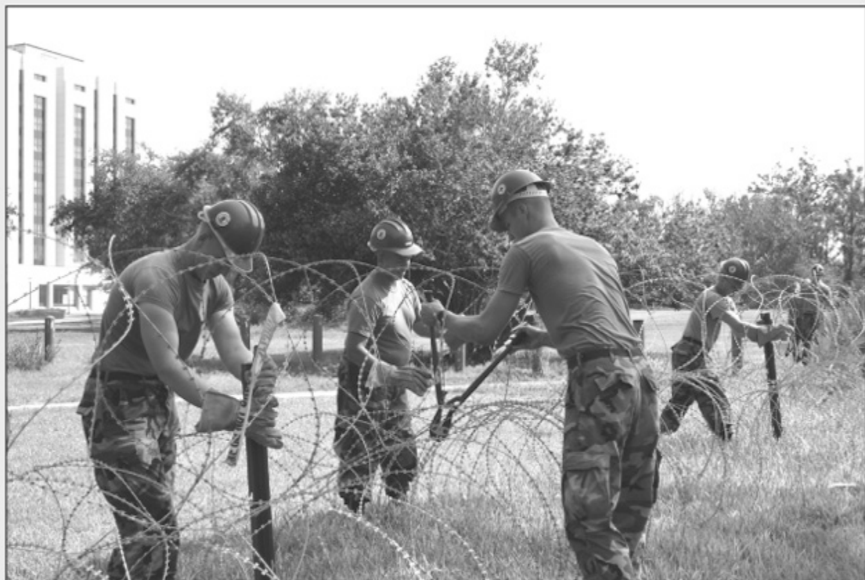
A hot job - Working in 95-100 degree temperatures, Seabees waste no time in getting the old fence down.
