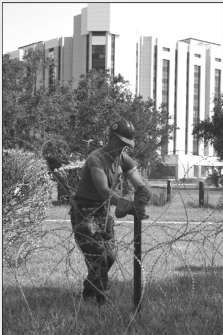
A Seabee pulls out of fence post in front of the AFRH.
