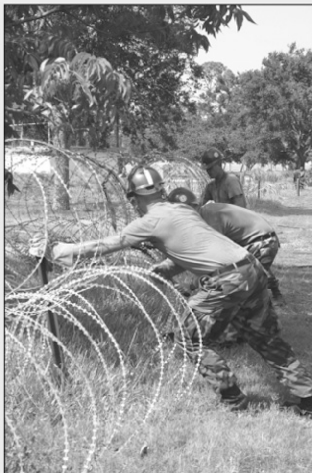
Several Seabees work along the front of the AFRH property cutting and rolling the existing wire to remove it.
