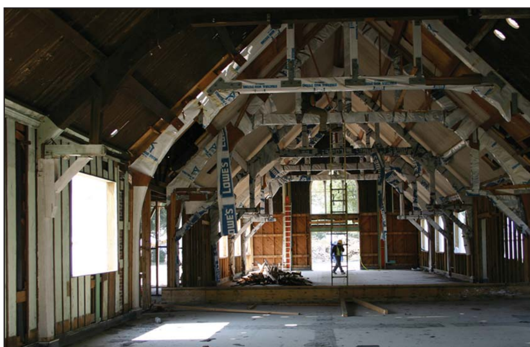
A construction contract for rehabilitation services of the Chapel was recently awarded. A crew is now onsite. Go to www.afrh.gov for more photos of the progress.
