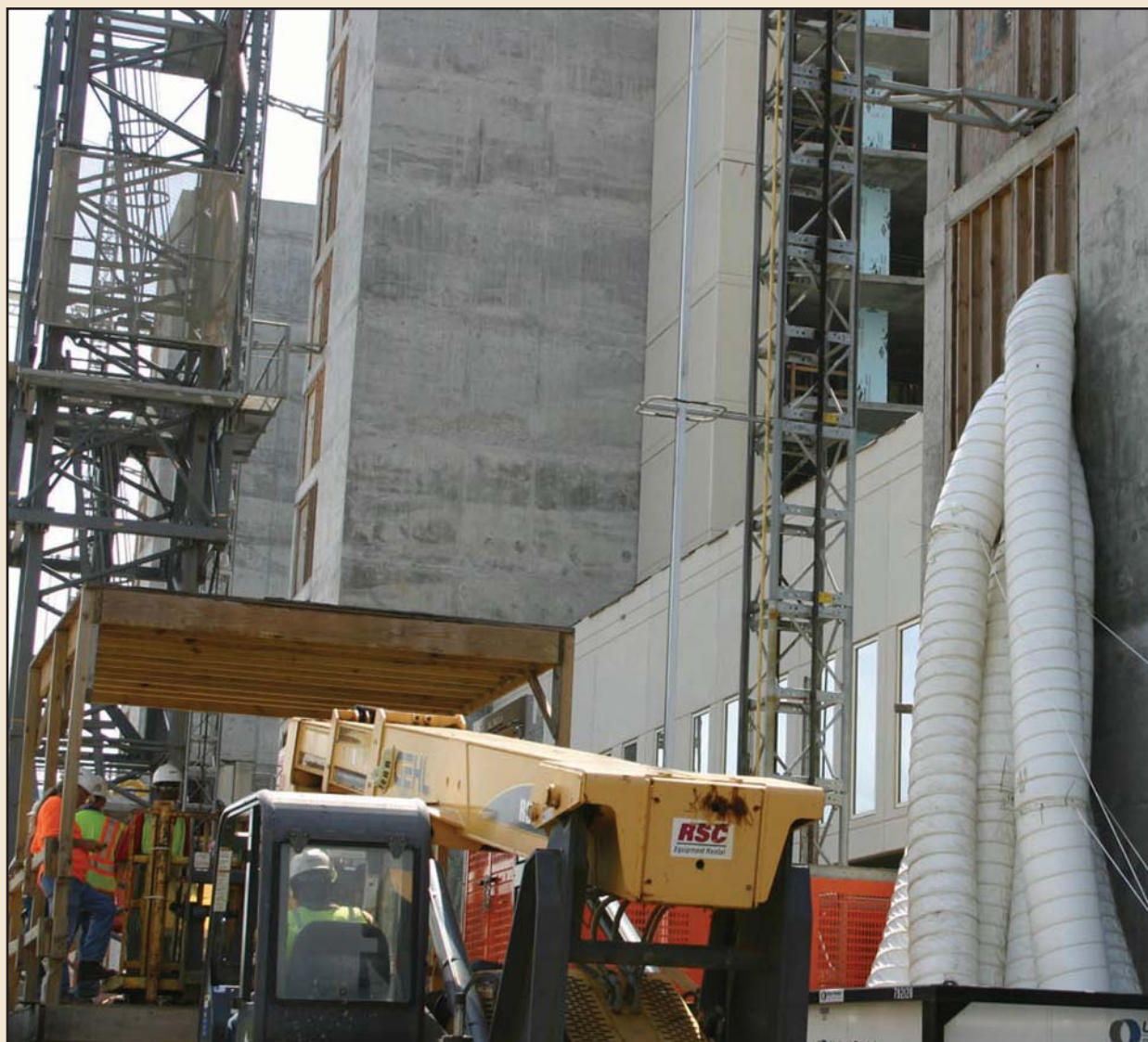
Pumping air - this is the north side of Towers C and B. As sheetrock work begins on the inside, these large white tubes are used to dehumidify the air.
