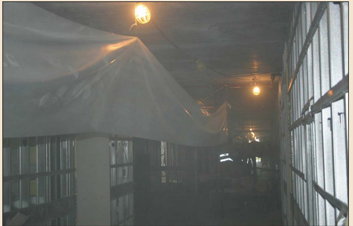
Dirty work - this is the hallway, north end looking south, on the 2nd floor of Tower A.
