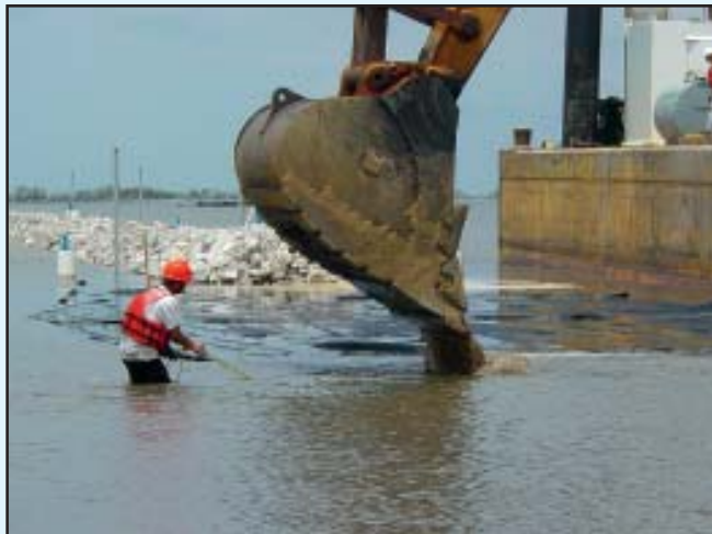
Placement of sand foundation on geotextile in native foundation displacement reach. (USACE)
