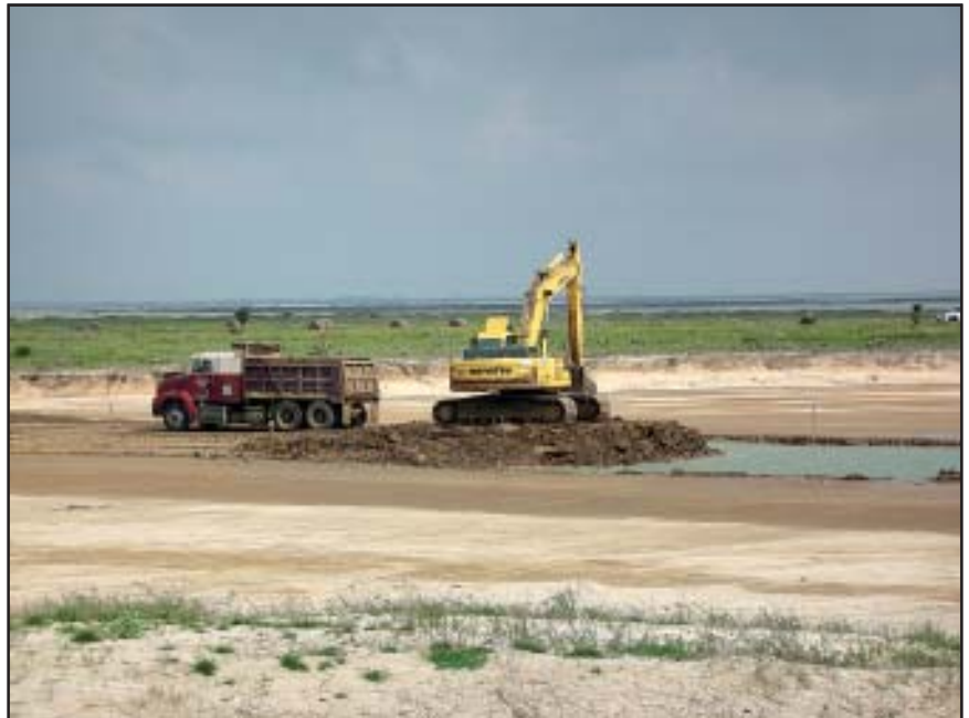
Heavy equipment operators remove excess material to create one of the channels connecting the three basins within the Babia Grande wetland complex, Texas. (Thor Lassen, Ocean Trust)
