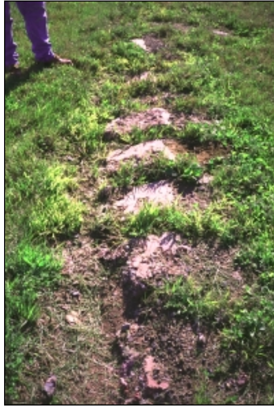
Figure 5-6. Typical erosion trough 16 months after SACON installation.
