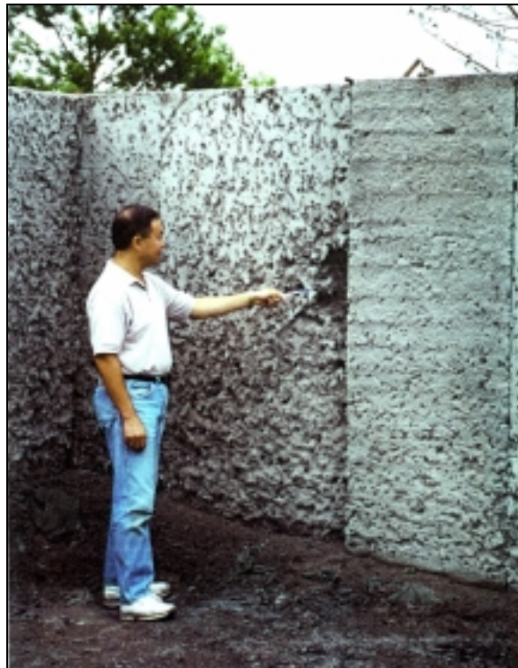
Figure 2-1. Live-Fire Training Facility using SACON.
