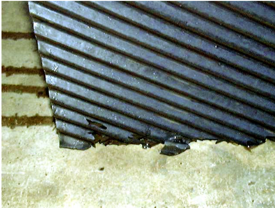
Figure 2.2-6. Location B, damaged coalescing plate.
