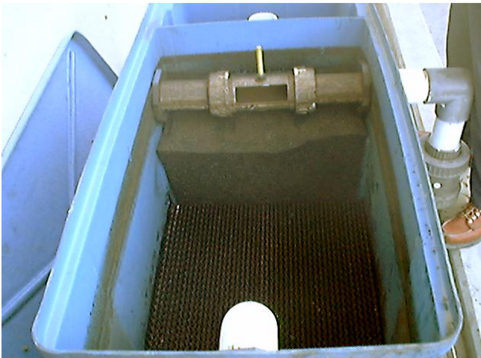
Figure 2.2-5. Location B, oil/water separator, top view, one coalescing plate package removed.
