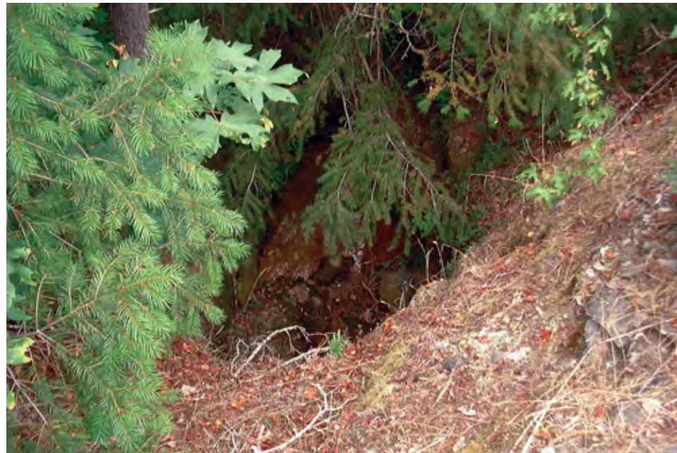
Figure A22. Hunts Hill drainage tunnel outlet, near Buckeye Ford in Greenhorn Creek, Nevada County, California.
