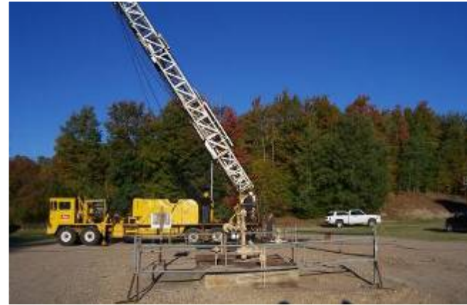
Monitoring Well (about 500 feet from injection well)
