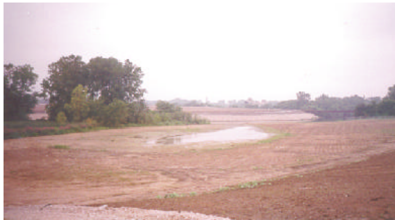
Low-lying area looking north toward the Ottawa River several weeks after completing remedial activities.
