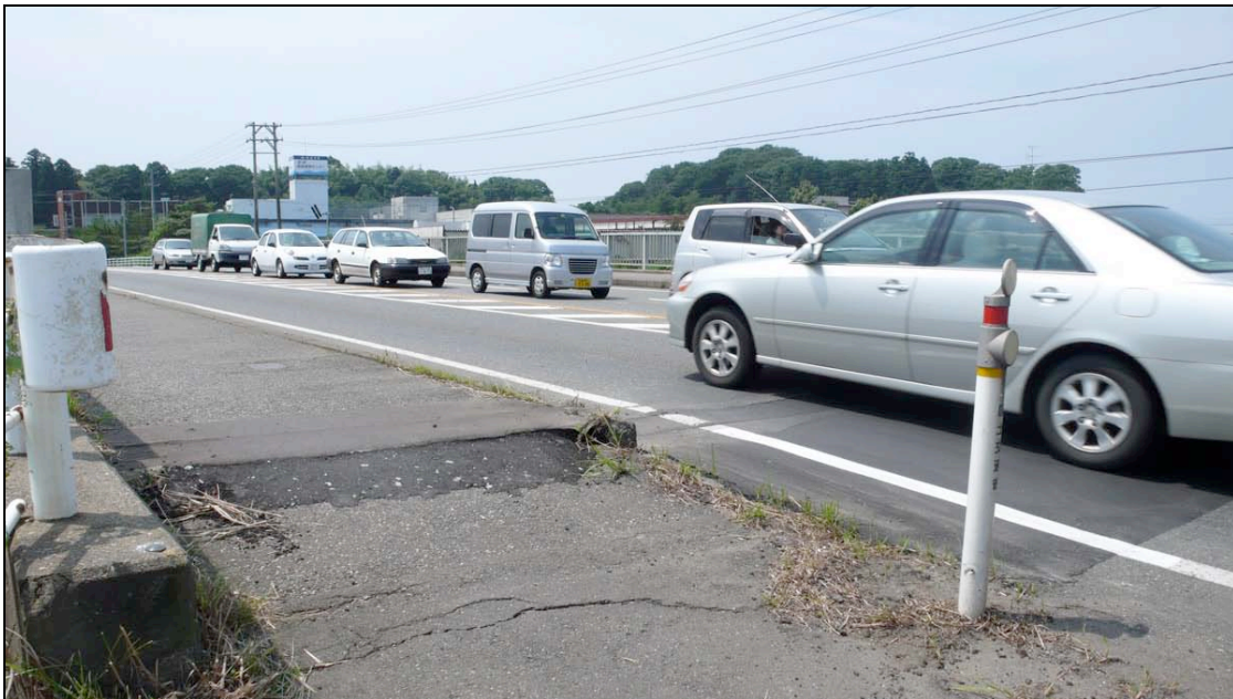
Fig. 6.19. Slight (10cm) settlement at bridge approaches.
