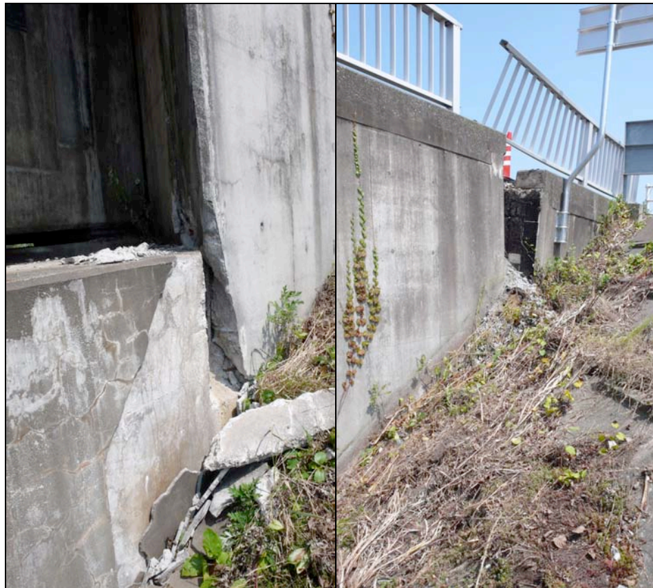
Fig. 6.51. Abutment and wingwall damage from the earthquake.
