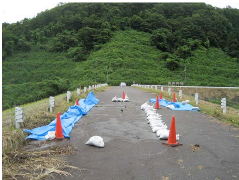
Figure 3.9: Embankment cracking and settlement of South Dam near Miyamo Parking Area along Highway 8, Nagaoka-Shi region (Site RK50; N37.43267° E138.73674°, photos taken 7/23/07 at approximately 11:15). The dam is a 15-meter tall, 97.5-meter wide earth fill structure with 3(H):1(V) downstream and 3.5(H):1(V) upstream benched slopes. Crest elevation is 63 meters and normal pool elevation is 55 meters. Observations were made of an embankment slope failure along the crest of this dam, through half the crest width (~4 m). Settlement and deformation occurred along a 10 m long section with up to 4 cm each of lateral and vertical deformation in the down slope direction. Contour-parallel ground cracking (2-4 cm wide, 1-2 m long) along the ground-spillway interface were also observed, two-thirds of the way down the dam face. The reservoir was empty and appeared to not have been filled in some time judging by the height of vegetation growing in the reservoir area.
