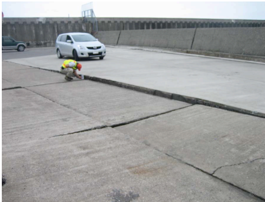
Figure 4.18: Kashiwazaki Harbor - South area experienced ground damage from liquefaction induced lateral spreading and settlement of separated pier slab sections (Site RK25, N37.36713° E138.53210°, 7/20/2007).
