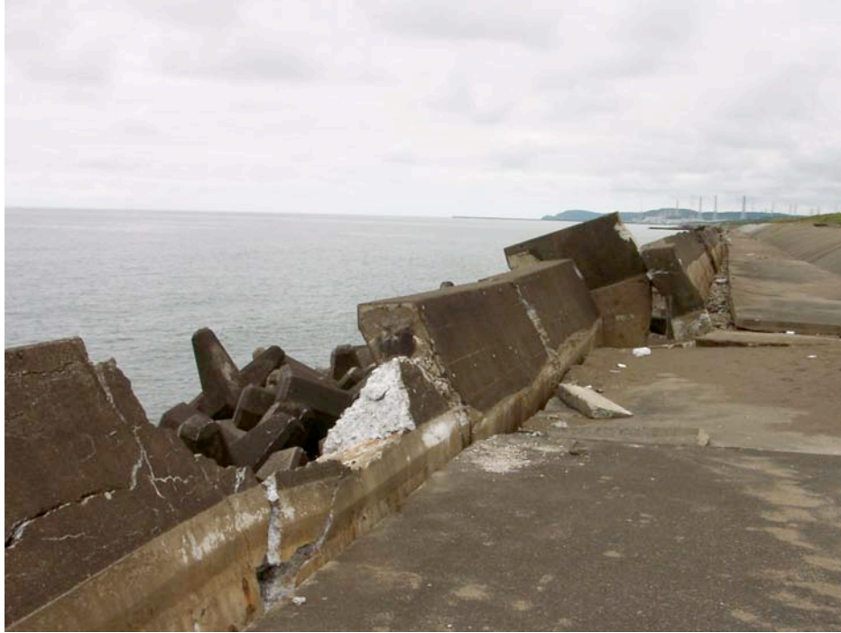
Figure 8.39: Lateral displacement, rotation, and structural damage to the seawall (Location is southwest of Site SD1, photo taken 7/22/07 11:45).
