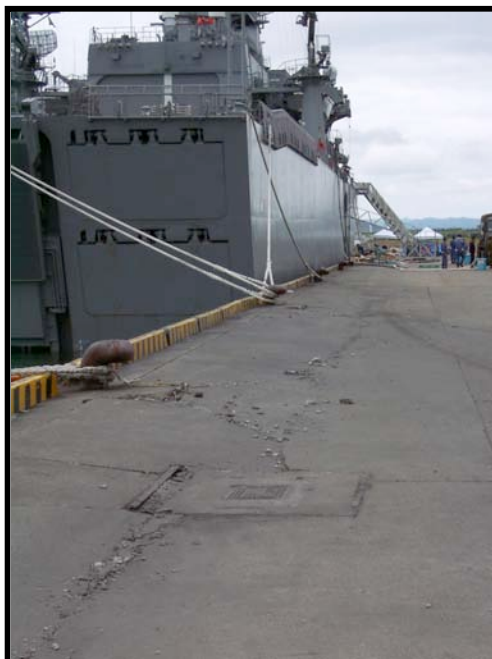
Figure 8.25: Kashiwazaki Port - Evidence of very minor lateral movement of quay walls and minor settlement located along the northern face of the terminal used as the berth for the Japan Self Defense Force (Site SD8, approximately N37.36680° E138.53825°, photo taken 7/22/07 15:24).
