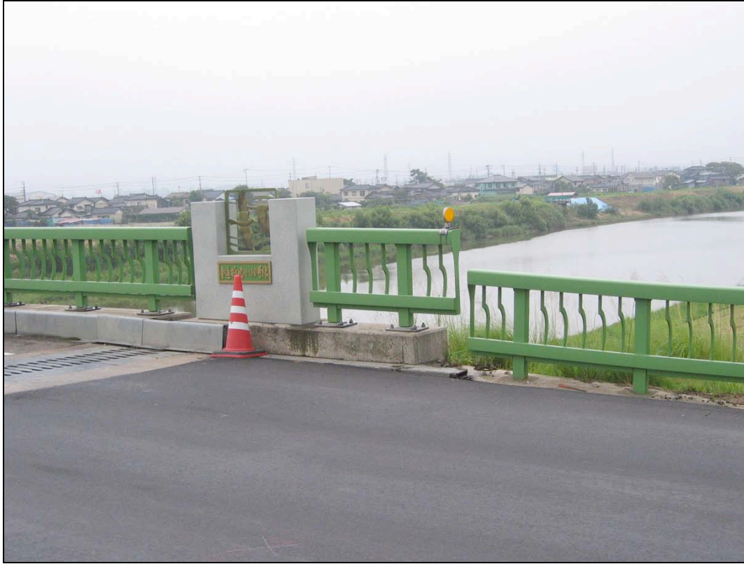
Fig. 6.35. Settlement of north bridge approach.
