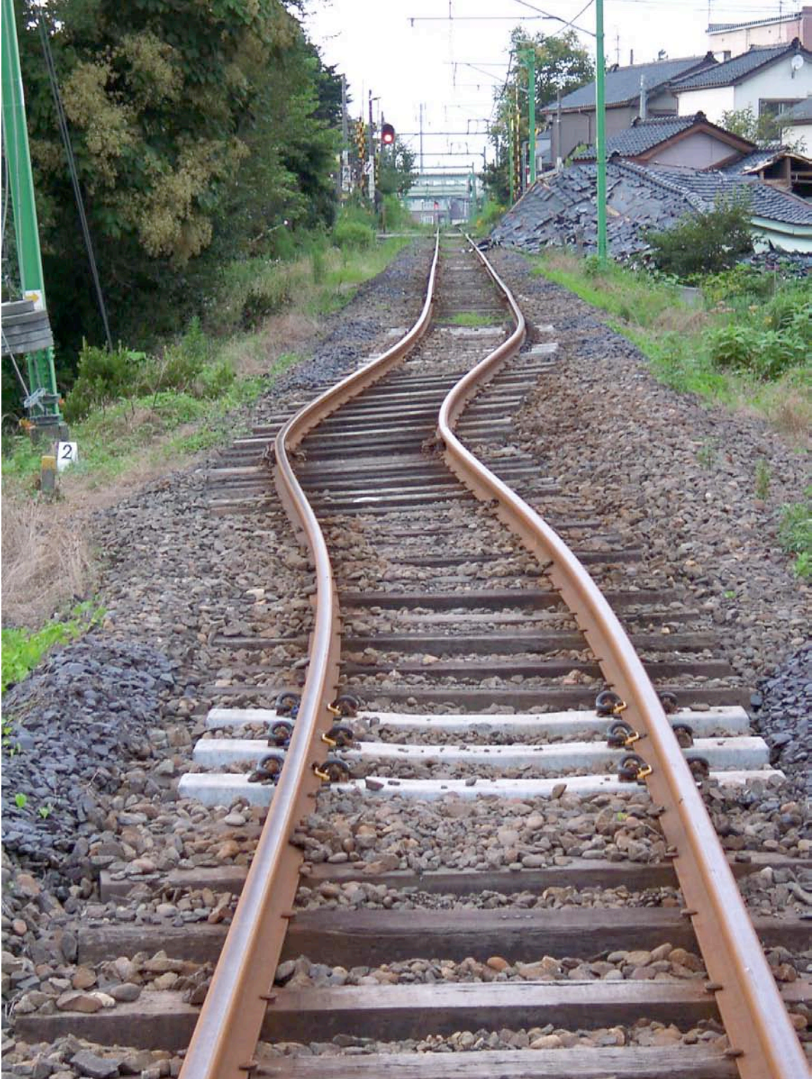
Figure 9.13: Lateral railway buckling (Site RK28, N37.37037° E138.56475°, 7/21/07 18:01).
