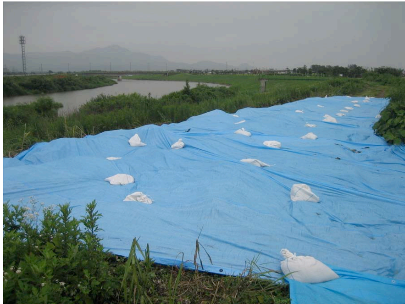
Figure 4.5: Kai-Un Bridge over Sabaishi River (Site RK4 N37.39233° E 138.58063°, 7/19/2007, 1:40 p.m.). Liquefaction induced crest cracking on the levee embankment near the northwest side of the bridge.
