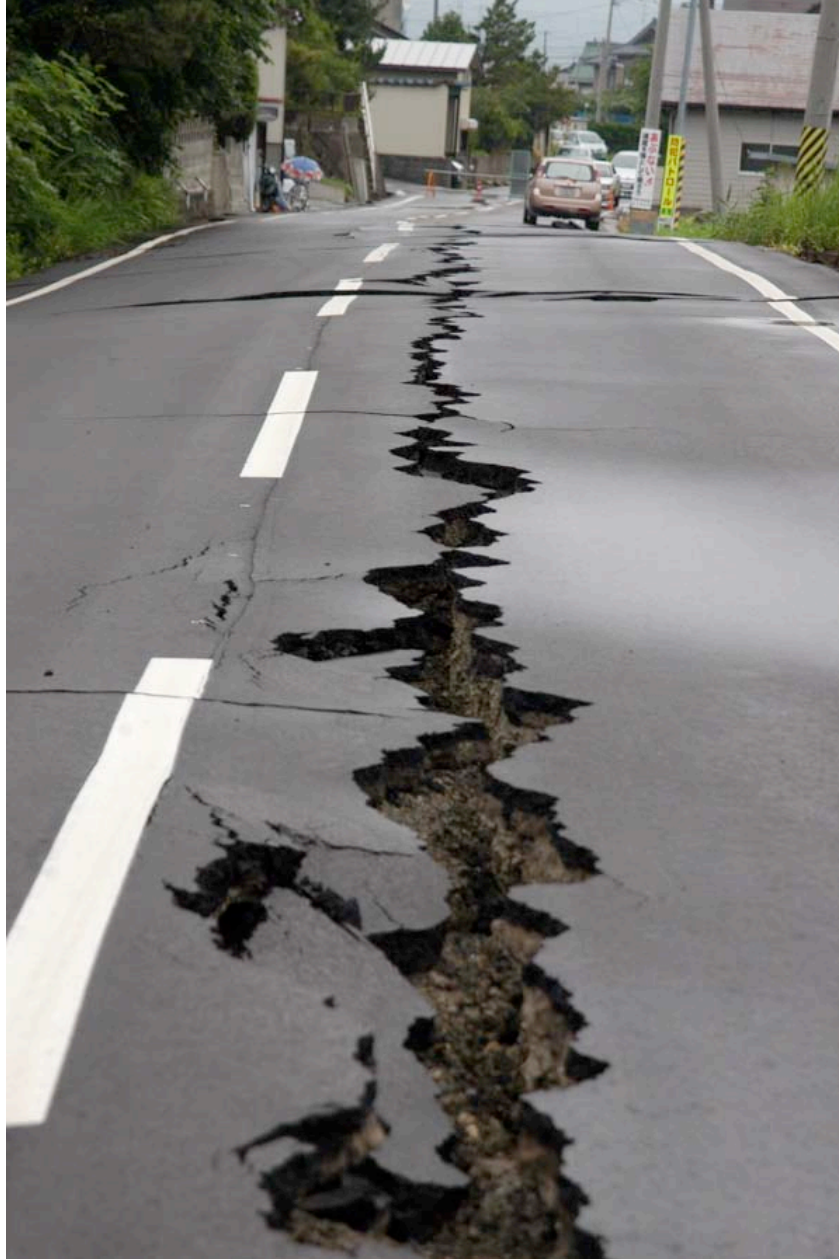
Figure 4.13: North side of Kai-Un Bridge area Sabaishi River - Lateral Spread on Road to Kashiwazaki Incinerator (Site RK6, N37.39343° E138.58555°, 7/19/2007). Lateral spreading on the north side of the river adjacent to the Kashiwazaki Municipal Incinerator damaged the access road of the facility.
