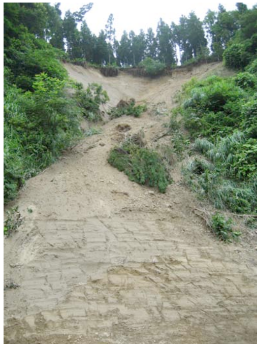
Figure 3.7: Ozumi-Mishimayamachi Landslides (Site RK2/YT2; N37.44057° E138.70467°, photos taken 7/20/07 at approximately 11:30). These slides occurred on a native hill slope and consisted of debris slumps in mudstone/siltstones and colluvium materials. High-resolution, topographic data was collected of these landslides using the terrestrial LiDAR scanning method.
