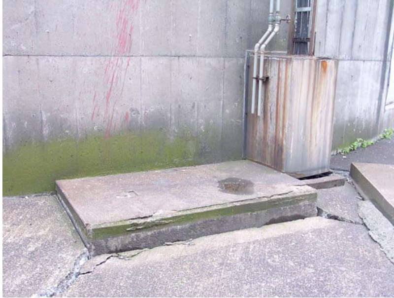
Figure 8.29: Kashiwazaki Port (Taiheiyo Cement Facility) - Evidence of minor to moderate settlement of sandy fill adjacent to one of the large diameter tanks (Site SD9, approximately N37.36665° E138.53983°, photo taken 7/22/07 15:48).
