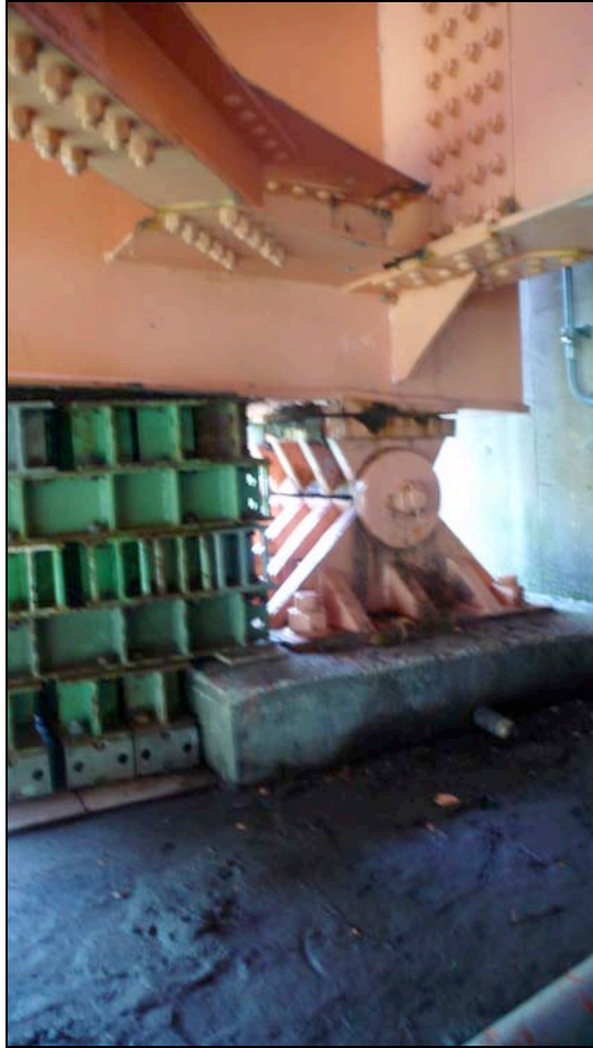
Fig. 6.27. Damage of set bolts and the additional steel box support to prepare the aftershocks)
