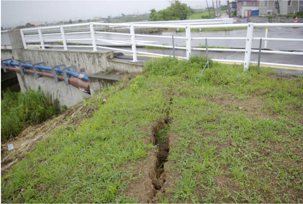
Figure 10.9: Evidence of moderate ground failure in an approach fill. Minor damage to the pipes was observed (Site RK7, N37.38940° E138.57393°, photo taken 7/21/07).
