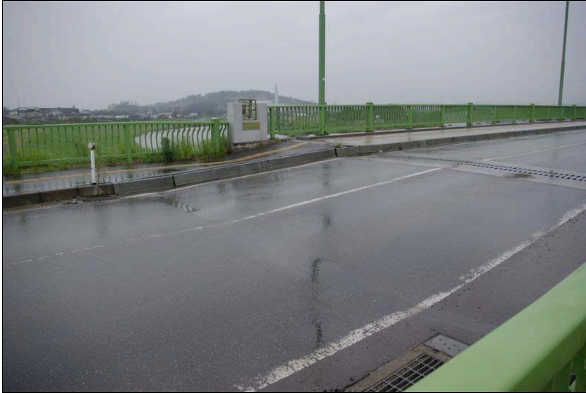
Fig. 6.39. Settlement of north bridge abutment.
