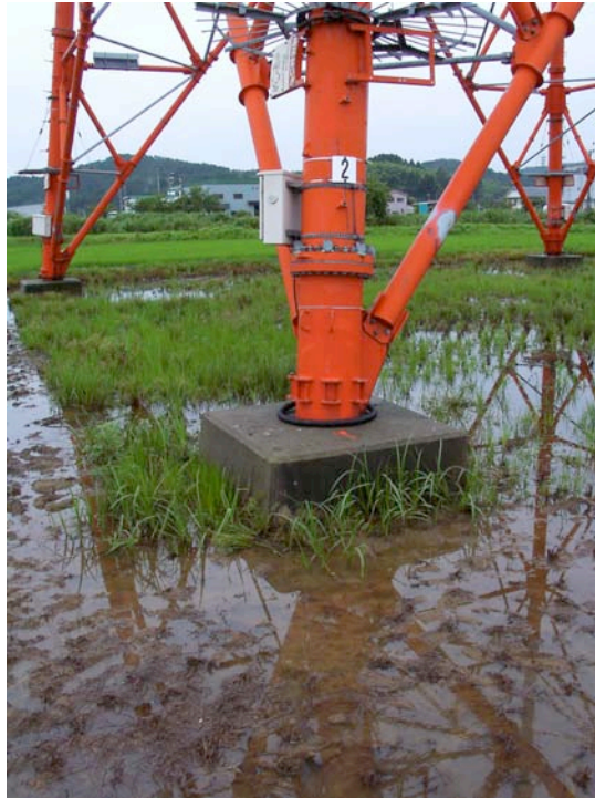
Figure 10.7: High voltage power line towers located in an area of soft ground (Site RK12, N37.44113° E138.63390°, photo taken 7/21/07). No evidence of ground failure, settlement, or structural damage to the towers was observed.
