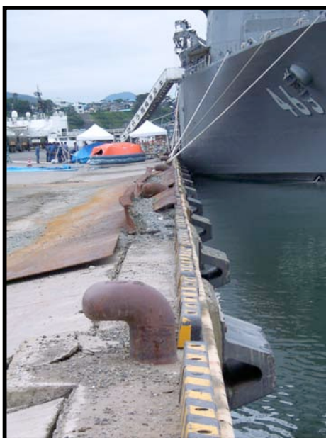
Figure 8.26: Kashiwazaki Port - Evidence of more extensive lateral caisson displacement and ground settlement adjacent to the quay wall located along the eastern end of the north face of the terminal (Site SD8, approximately N37.36680° E138.53825°, photo taken 7/22/07 15:36).
