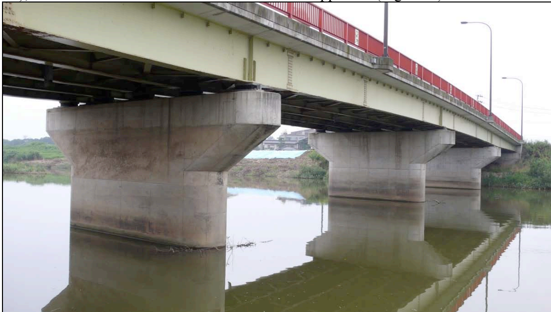
Fig. 6.40. The four, steel 'I' girder span Kaiun Bridge on pier walls and seat abutments.
