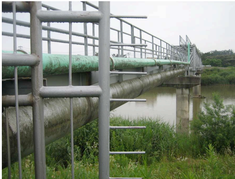
Figure 4.3: Kai-Un Bridge over Sabaishi River (Site RK4 N37.39233°,E 138.58063°, 7/19/2007, 1:40 p.m.). A water pipeline rupture was found with pipe offsets of 13 cm in the horizontal direction, 10 cm in the vertical direction, and with 40 cm of associated nearby settlement between the pipeline and the ground.
