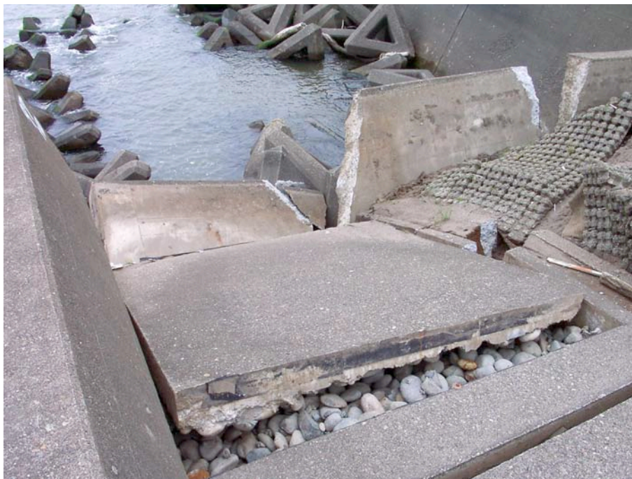
Figure 8.34: Close-up of the collapsed portion of the seawall showing the clean cobble backfill (Site SD1, N37.38868° E138.56413°, photo taken 7/22/07 11:23).
