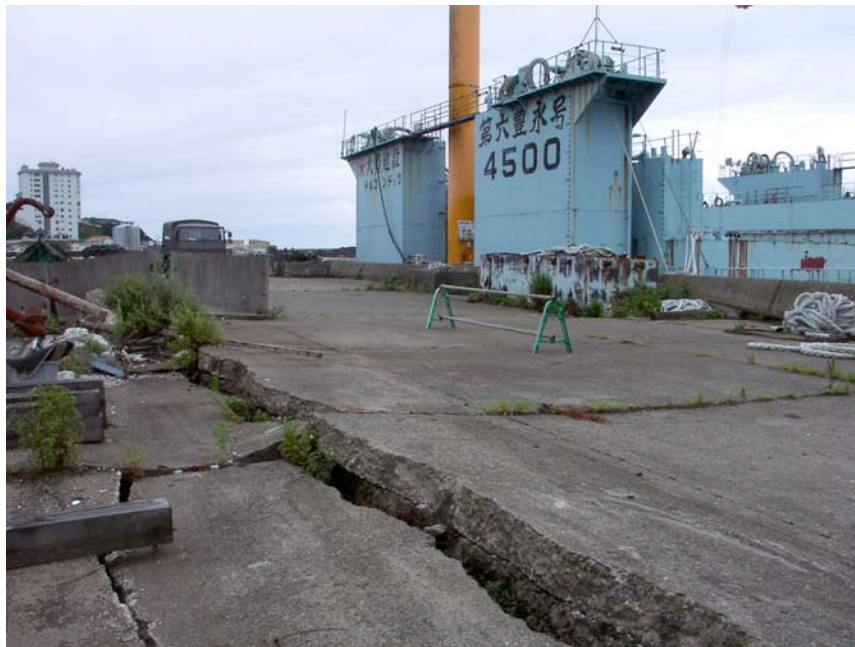
Figure 8.19: Kashiwazaki Port - Steel Scrap Transport Facility showing evidence of ground failure due to liquefaction of sand fill and damage to concrete aprons (Site SD6, N37.36668° E138.53565°, photo taken 7/22/07 14:46).
