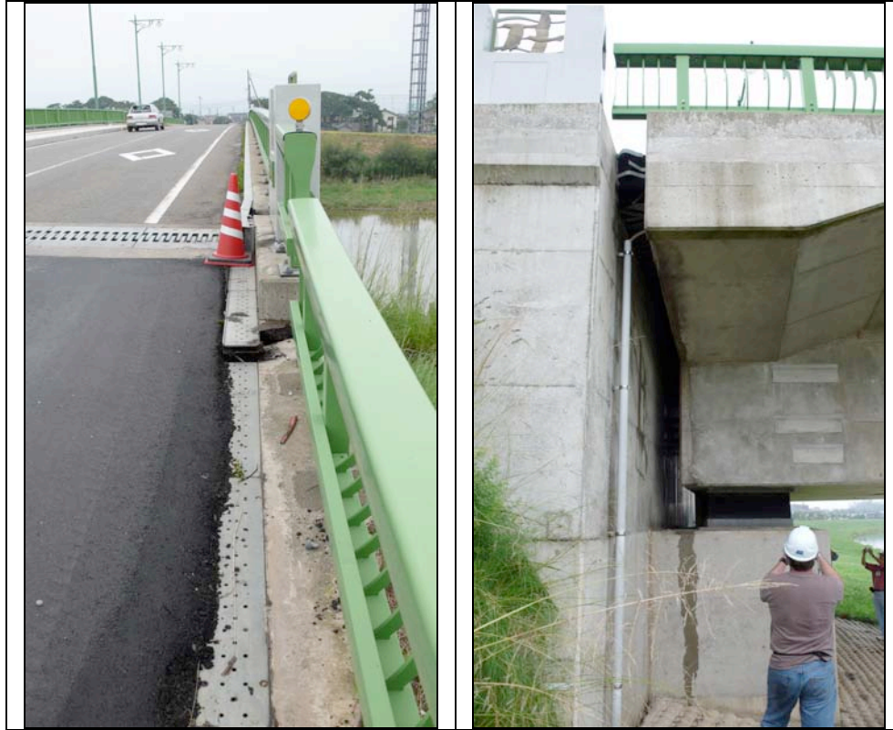
Fig. 6.37. Signs of movement of the abutments included distortion of bearings.
