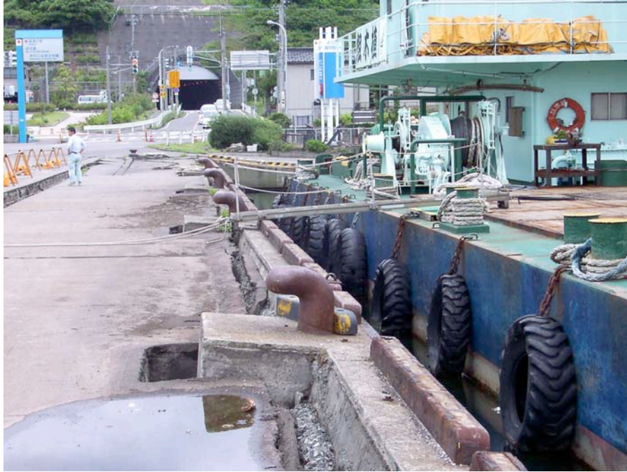
Figure 8.16: Kashiwazaki Port - West facing portion of the “Southwestern Pier” showing displacement of the sheet pile wall and ground settlement due to liquefaction of sandy backfill (Site SD5, N37.36532° E138.53213°, photo taken 7/22/07 13:57).
