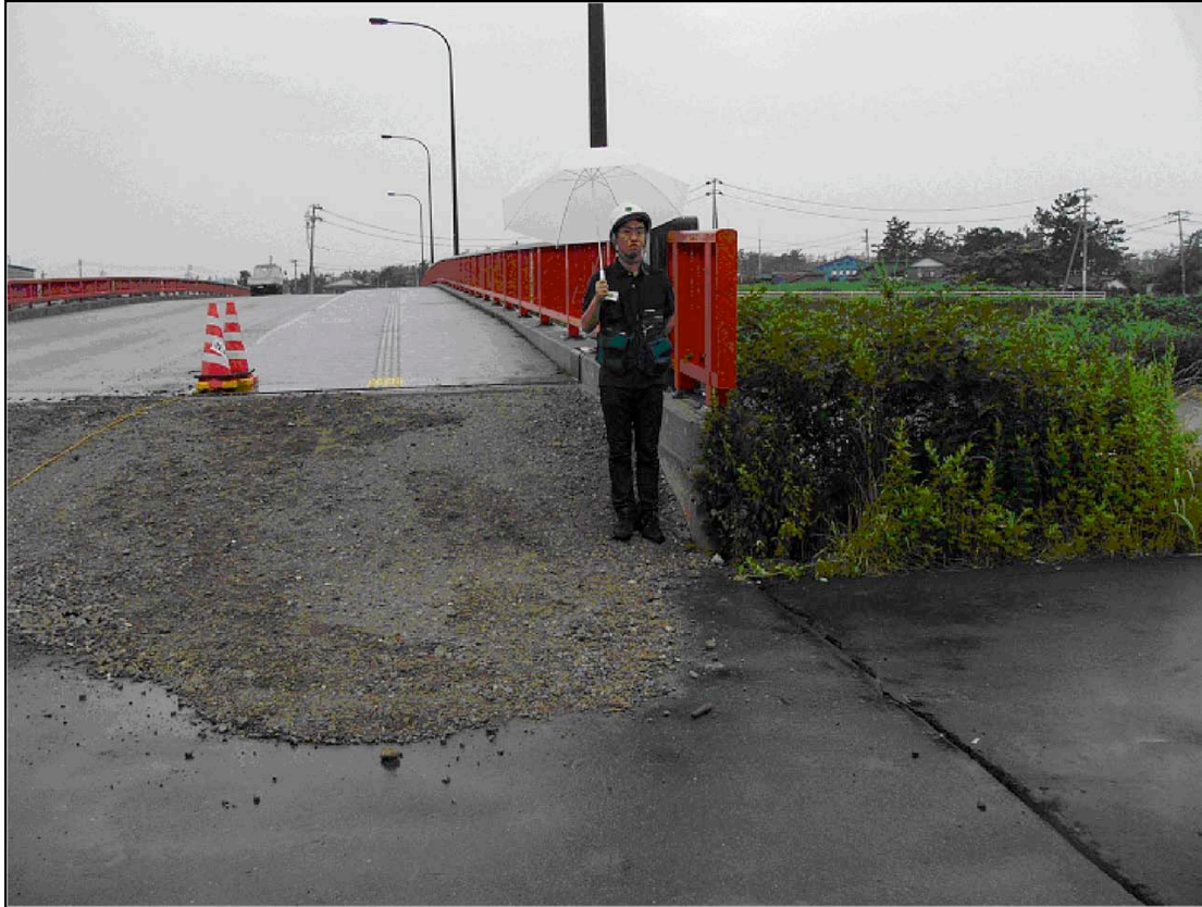
Fig. 6.41. About one meter settlement of south Kaiun bridge approach.
