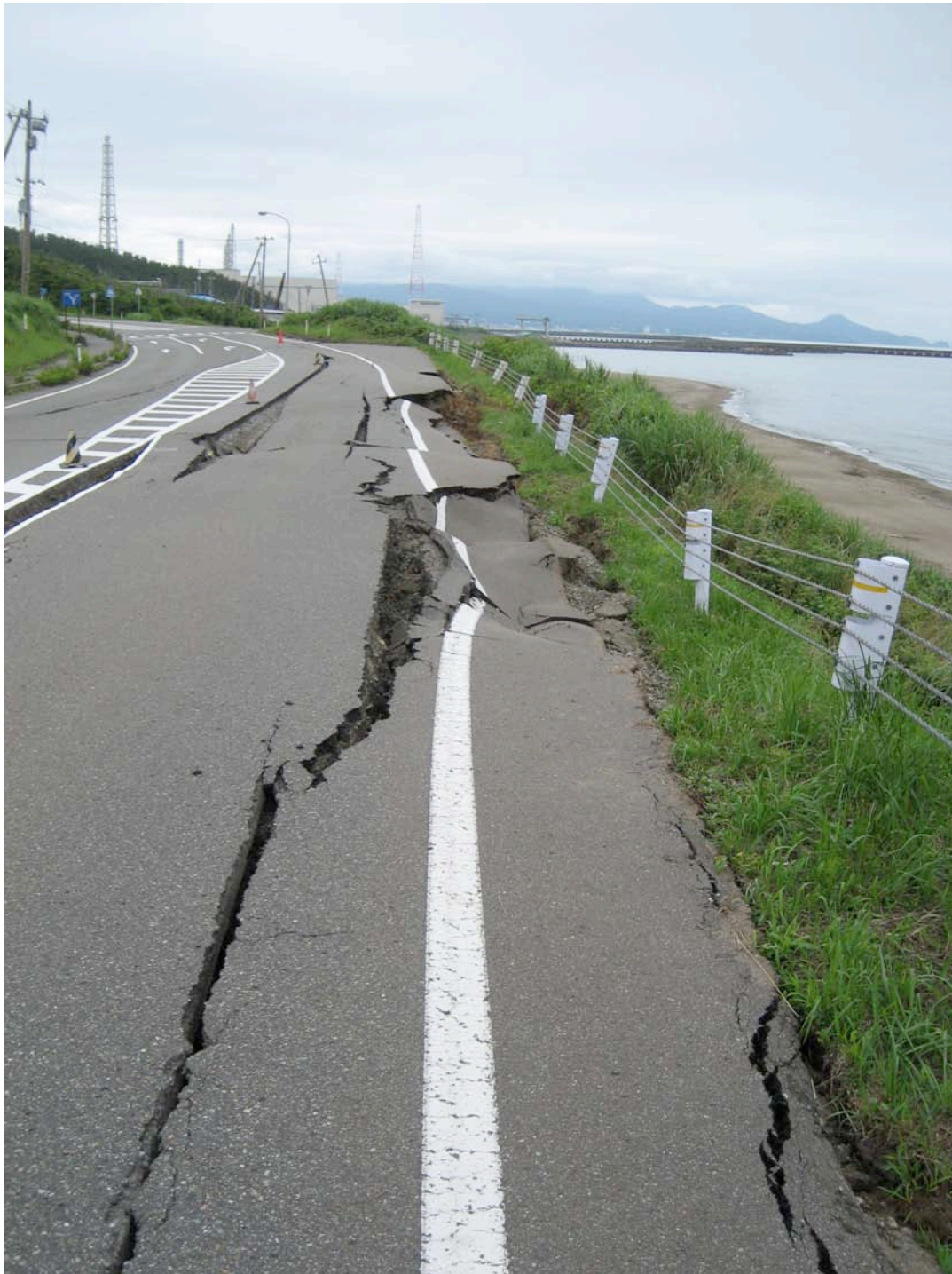
Figure 9.3: Road damage from fill embankment failure on coastal road north of Kashiwazaki Nuclear Power Station (Site RK38, N37.44927° E138.60572°, photo taken 7/22/07 13:04). Such damage tended to increase with distance toward the epicenter, often requiring traffic controls to guide cars across the one open lane.
