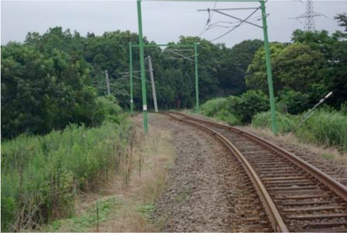
Figure 9.14: Vertical deformation in train tracks (Site SA24, N37.39323° E138.59520°, 7/21/07 15:44).
