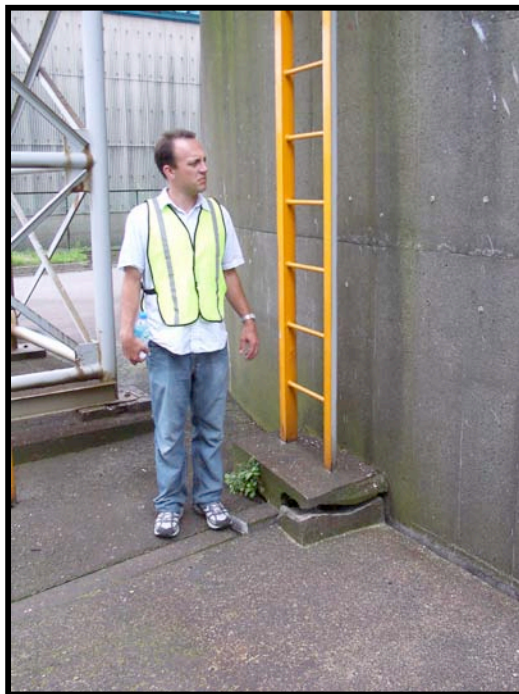
Figure 8.30: Kashiwazaki Port (Taiheiyo Cement Facility) - Evidence of minor to moderate settlement of sandy fill adjacent to one of the large diameter tanks (Site SD9, approximately N37.36665° E138.53983°, photo taken 7/22/07 15:48).
