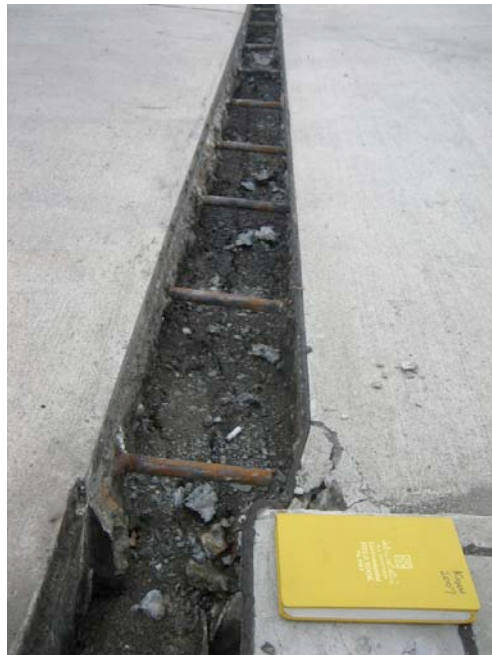
Figure 4.20: Kashiwazaki Harbor - South area experienced ground damage from liquefaction-induced lateral spreading resulting in separated pier slab sections (Site RK25, N37.36713° E138.53210°, 7/20/2007).
