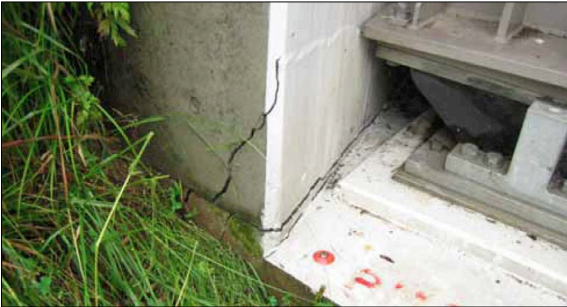
Fig. 6.46. Distorted bearing and cracked abutment backwall (photo courtesy of Scott Brandenburg).
