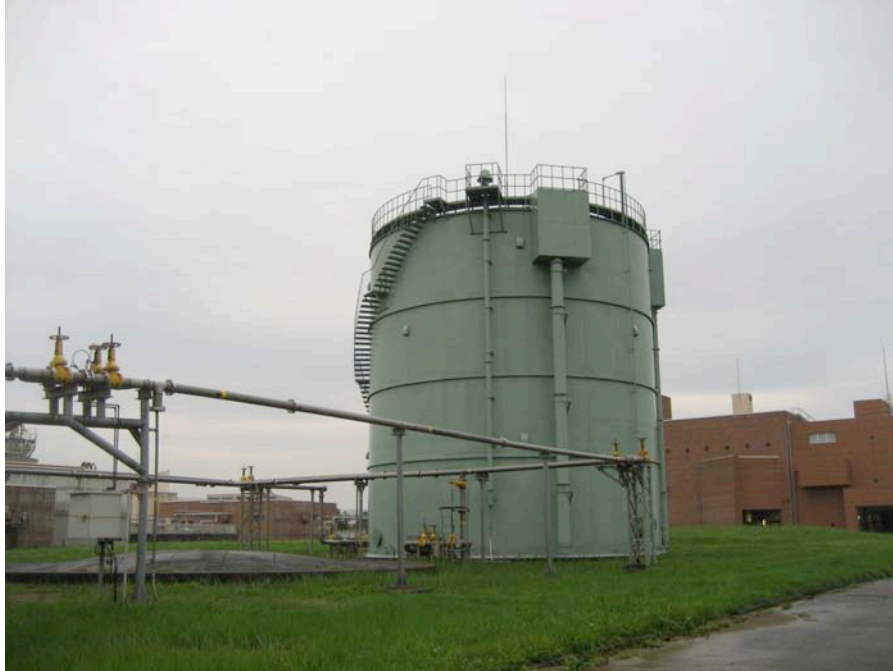
Figure 7.1: Steel tank at the Ansei-Chou waste water treatment plant (Site RK9, N37.38748°, E138.56587°, photo taken 7/20/07 16:40). Sand boils and slight overturning of the support member to the far-most right of the photograph were observed, as was extensive lateral spreading and road damage. Indications of minor distress of the tank was identified but for the most part appeared in good service.
