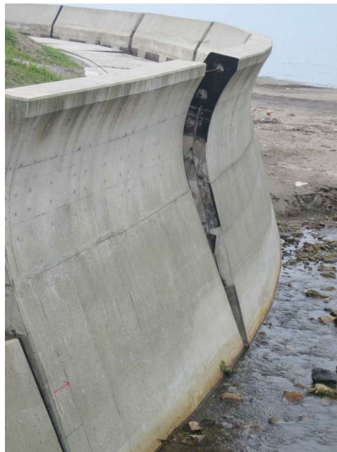
Figure 8.42: Rotation and lateral displacement of the concrete seawall (Site RK37, N37.45478°, E138.60927°, photo taken 7/23/07).
