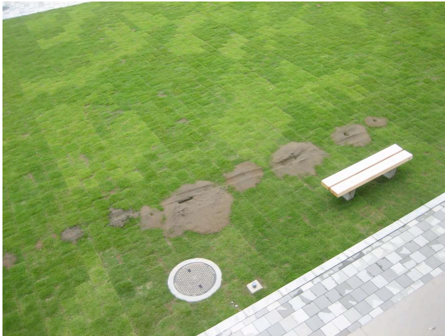
Figure 4.26: Kashiwazaki Harbor - South area exhibited surficial features of liquefaction on all sides of the port building. (Site RK25, N37.36713° E138.53210°, 7/20/2007).
