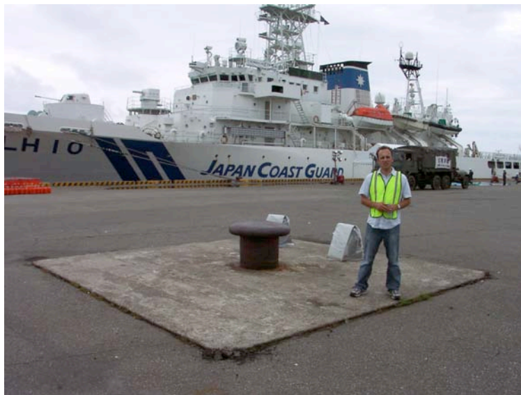
Photo 8.24: Kashiwazaki Port - Evidence of minor settlement adjacent to a pile-supported (?) bollard anchorage located along the northern face of the terminal used as the berth for the Japan Coast Guard (Site SD8, N37.36680° E138.53825°, photo taken 7/22/07 15:21).
