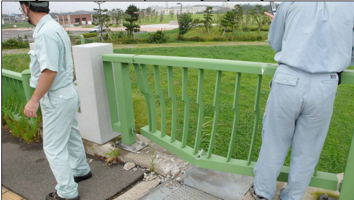
Fig. 6.38. Pounding between abutment and wingwall.
