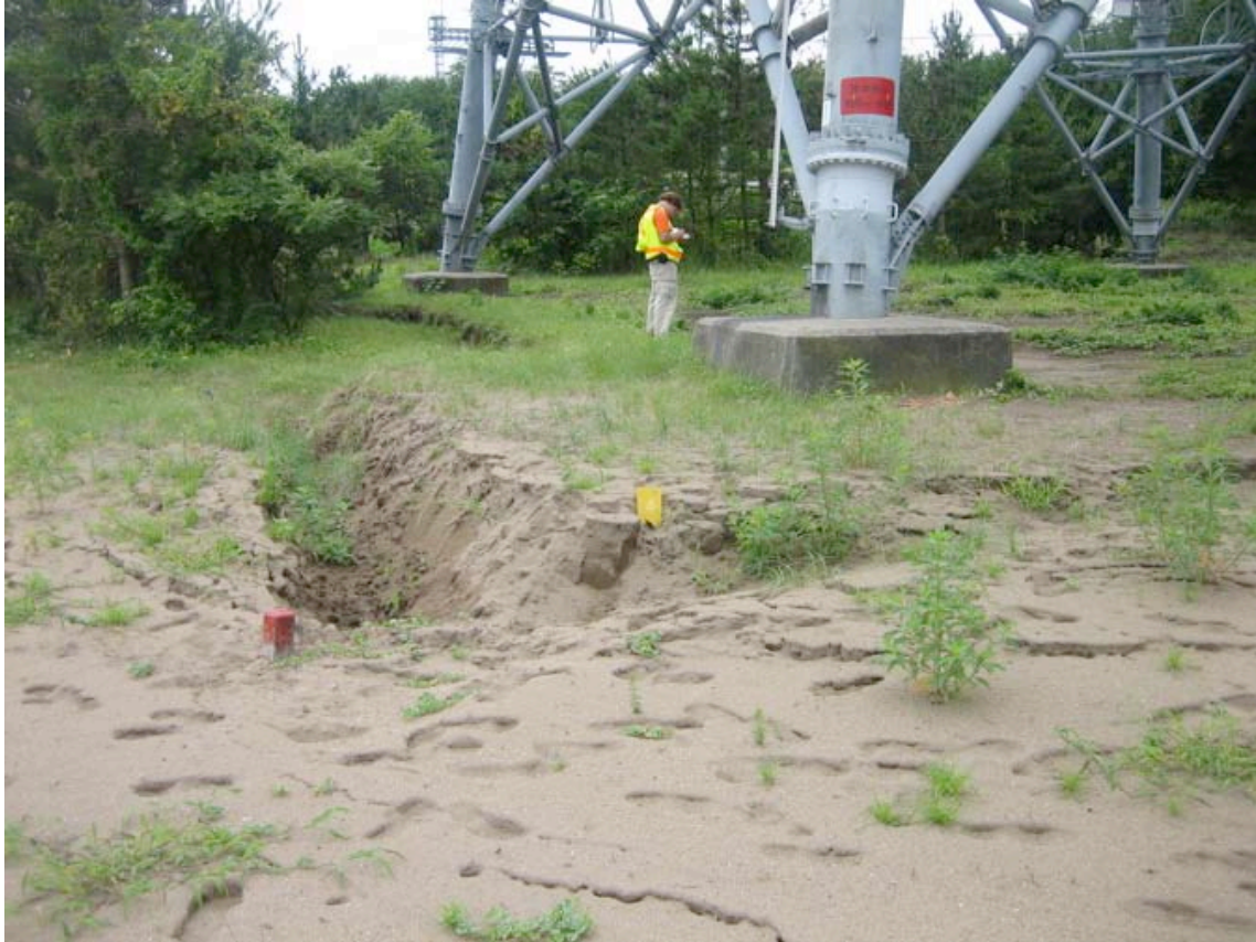
Figure 4.33: Liquefaction and lateral spread of ground adjacent to High Voltage Transmission Line Tower (Site RK40, N37.41633° E138.60792°, 7/22/2007).
