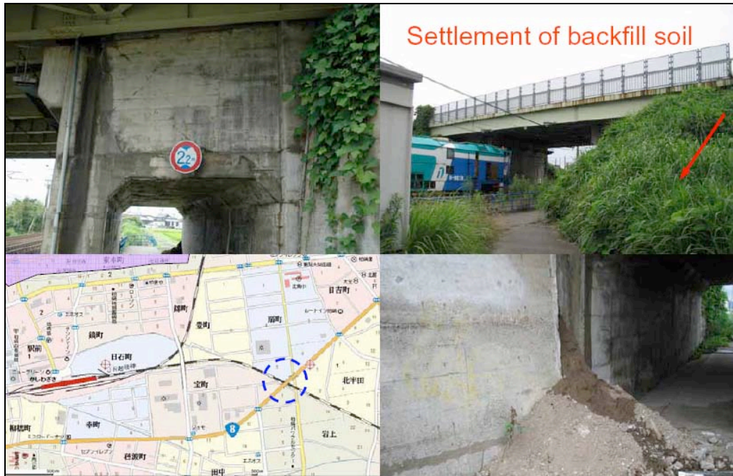
Fig. 6.17. Damage and repairs where railway crosses Highway 8 Bridge (courtesy G. Watanabe, Tokyo Institute of Technology).
