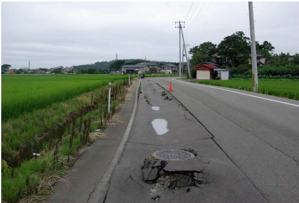
Figure 9.9: Pavement damage caused by utility trench liquefaction (Site SA21, N37.38950° E138.59662°, photo taken 7/21/07 14:57).
