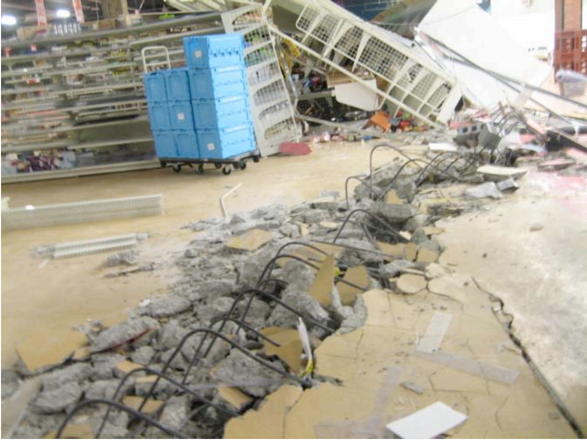
Figure 4.39: Plant 5 – Failure of slab on grade with buckled reinforcing bars. (Site RK41, N37.41468° E138.60840°, 7/22/2007).
