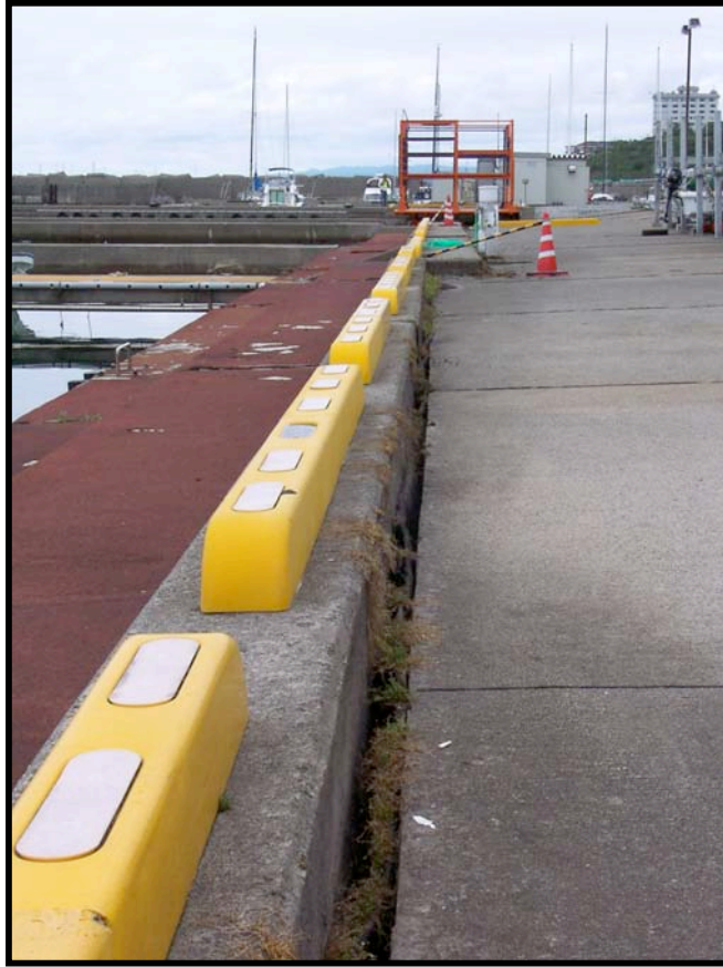
Figure 8.4: Kashiwazaki Marina - Evidence of minor lateral movement of quay walls and associated settlement of the paved apron (Site SD3, N37.36093° E138.52027°, photo taken 7/22/07 12:59).
