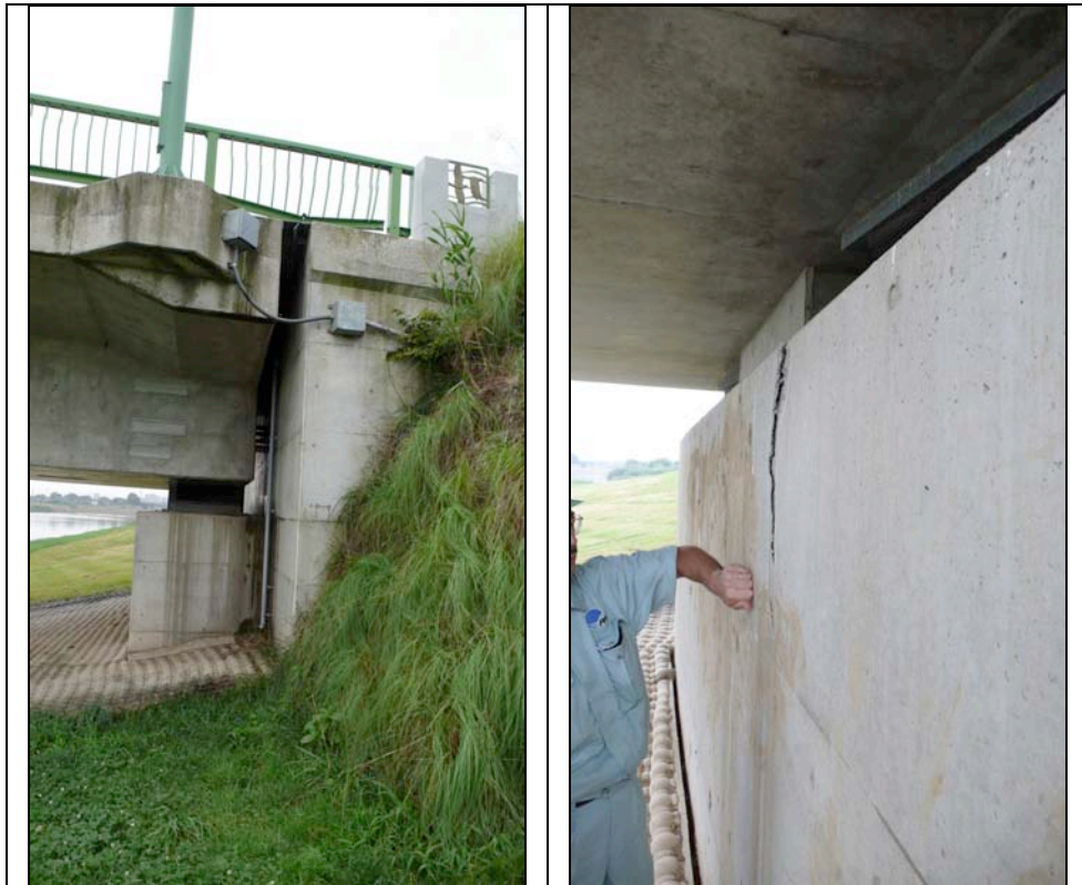
Fig. 6.36. The superstructure and bearings moved back and forth, cracking the abutment.
