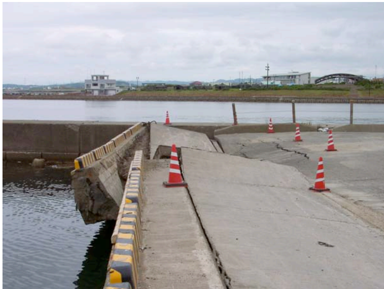
Figure 8.28: Kashiwazaki Port - Significant liquefaction-related damage to the quay walls located adjacent to the U River (Site SD8, approximately N37.36680° E138.53825°, photo taken 7/22/07 15:36).
