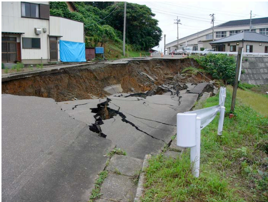
Figure 3.8: Road embankment failure off Route 8 on the way to Kasashima (Site YT18; N 37.33325 ° E 138.46500°, photos taken 7/21/07 at approximately 15:40). The slope appears to have undergone previous stabilization using slope grading and gabion baskets to support the toe.
