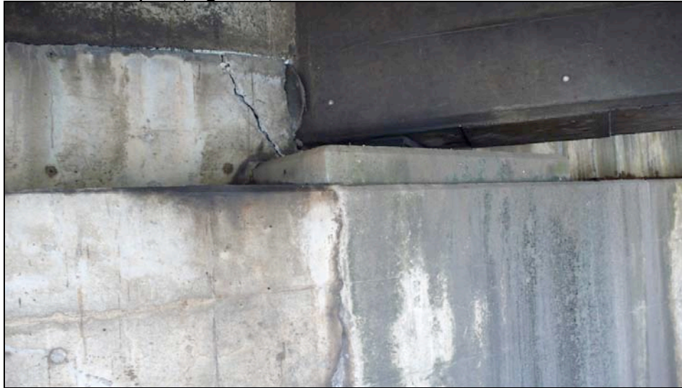
Fig. 6.52. Backwall-Diaphragm damaged by earthquake.
