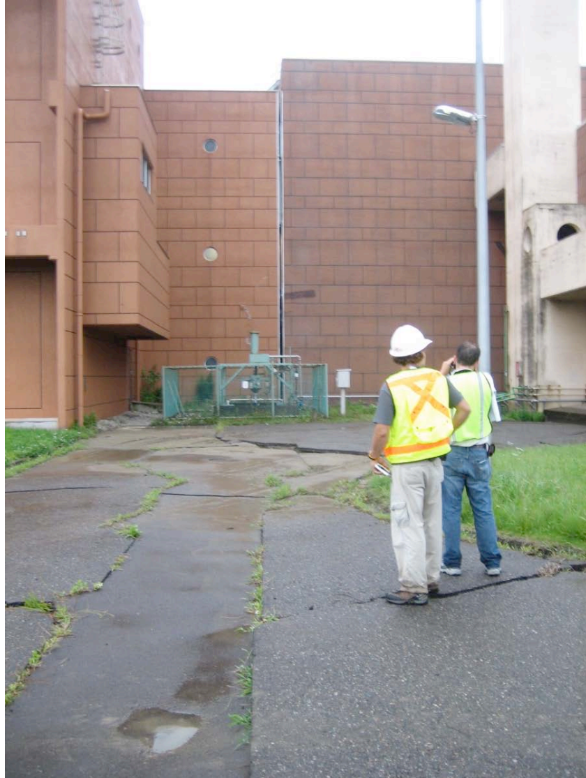
Figure 4.16a: Kashiwazaki Wastewater Treatment Plan on the south side of Sabaishi River near its outlet to the Sea of Japan (Site RK9 N37.38748° E138.56587°, 7/19/2007). Damage to the main building from liquefaction of ground resulted in the complete separation of two sections of the adjacent, yet integrated, three-story buildings with associated building and ground settlements.
