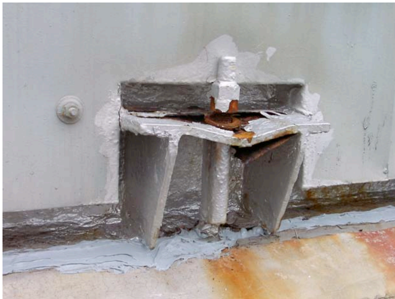
Figure 7.6: Kashiwazaki Port - Anchorage of asphalt storage tank (Located near Site RK25, N37.36713° E138.53210°, photo taken 7/22/07 12:37).
