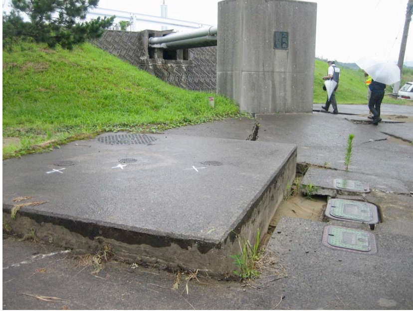
Figure 4.4: Kai-Un Bridge over Sabaishi River (Site N37.39233°, E138.58063°, 7/19/2007, 1:40 p.m.). A water cistern near the pipeline rupture uplifted in liquefied ground.
