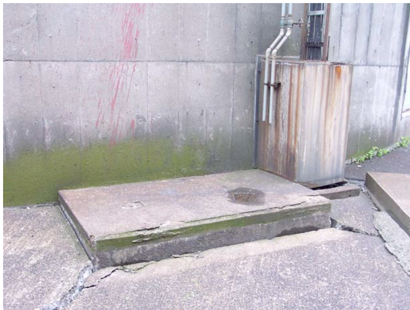
Figure 7.8: Kashiwazaki Port (Taiheiyo Cement Facility) - Evidence of minor to moderate settlement of sandy fill adjacent to one of the large diameter tanks (Site SD 9, approximately N37.36665° E138.53983°, photo taken 7/22/07 15:48).
