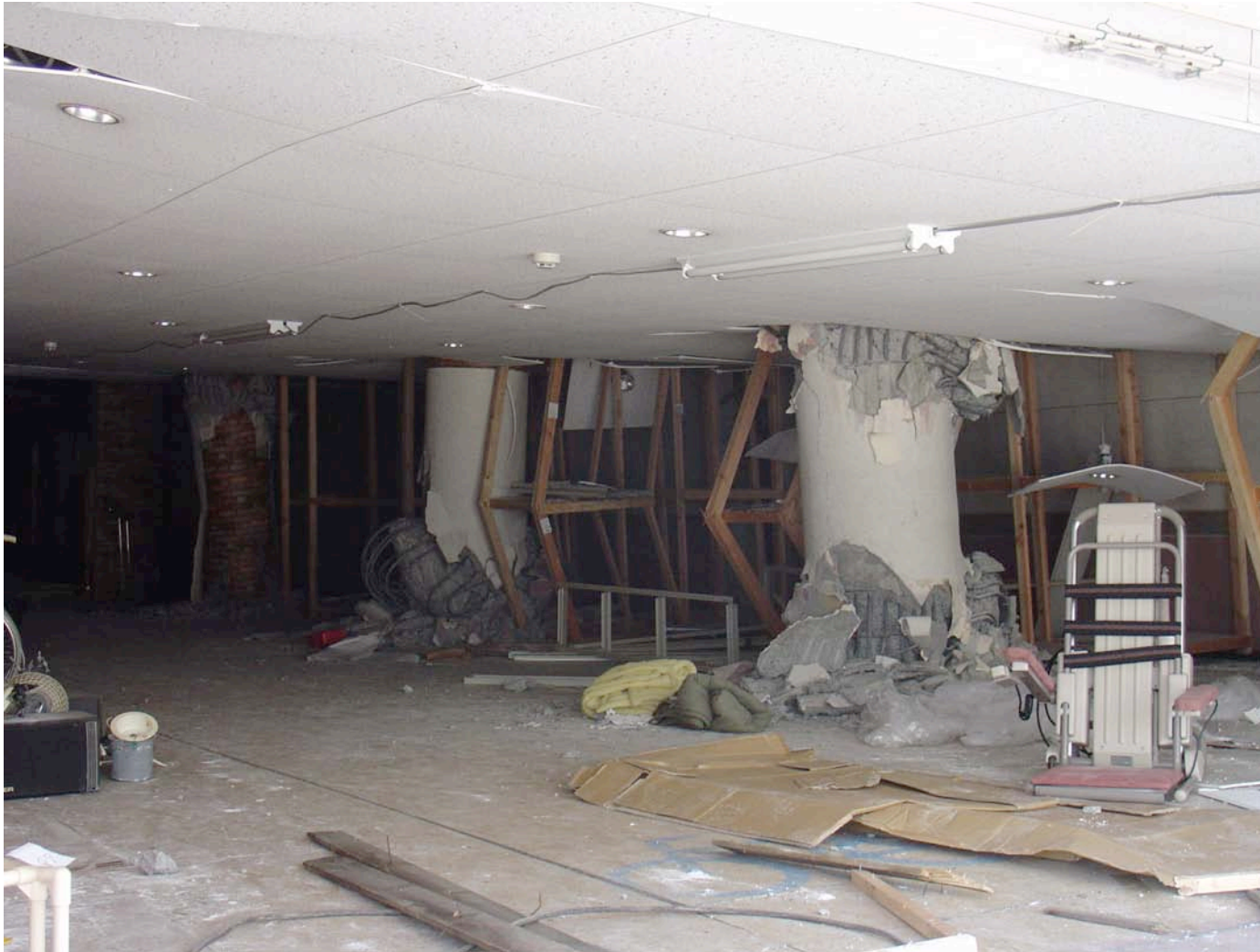
Figure 5.24: Shear failures of reinforced concrete columns (Site NIT-81, N37.37000° E13855825°, photo by Peter Yanev)
