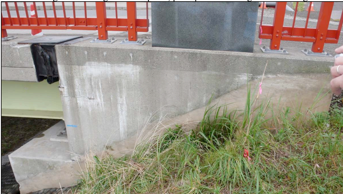
Fig. 6.42 The soil around the south abutment moved towards the river during the earthquake.
