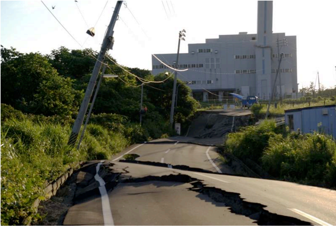
Figure 9.2: Road to Kashiwazaki municipal waste incinerator plant (Site RK6, N37.39343° E138.58555°, photo taken 7/24/07 18:06). Liquefaction-induced lateral spreading led caused the roadbed and associated slope to move southwards towards the Sabaishi River. Photos show formation of a 2.5 meter tall head scarp at the west end.
