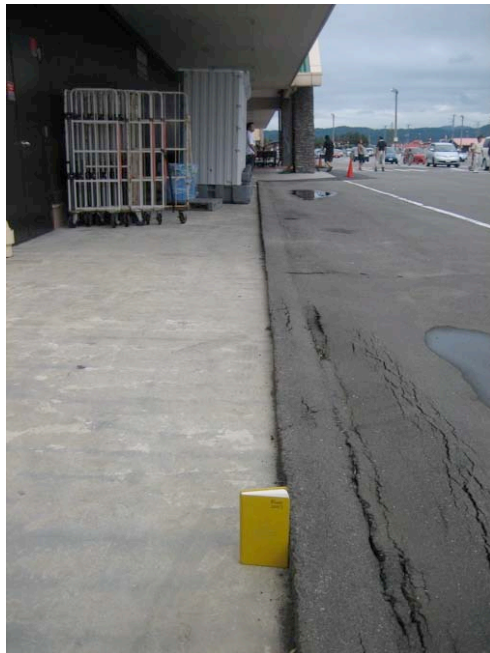
Figure 4.38: Plant 5 Store - Ground settlement in dune sand was observed around the building and an underground storage tank had been uplifted (Site RK41, N37.41468° E138.60840°, 7/22/2007).
