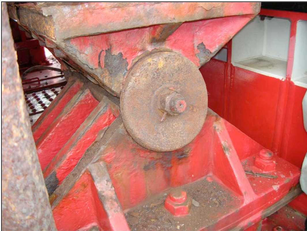
Fig. 6.23. Deformation of Bearing Pin-Cap caused by uplift force (courtesy of S. Unjoh, PWRI).
