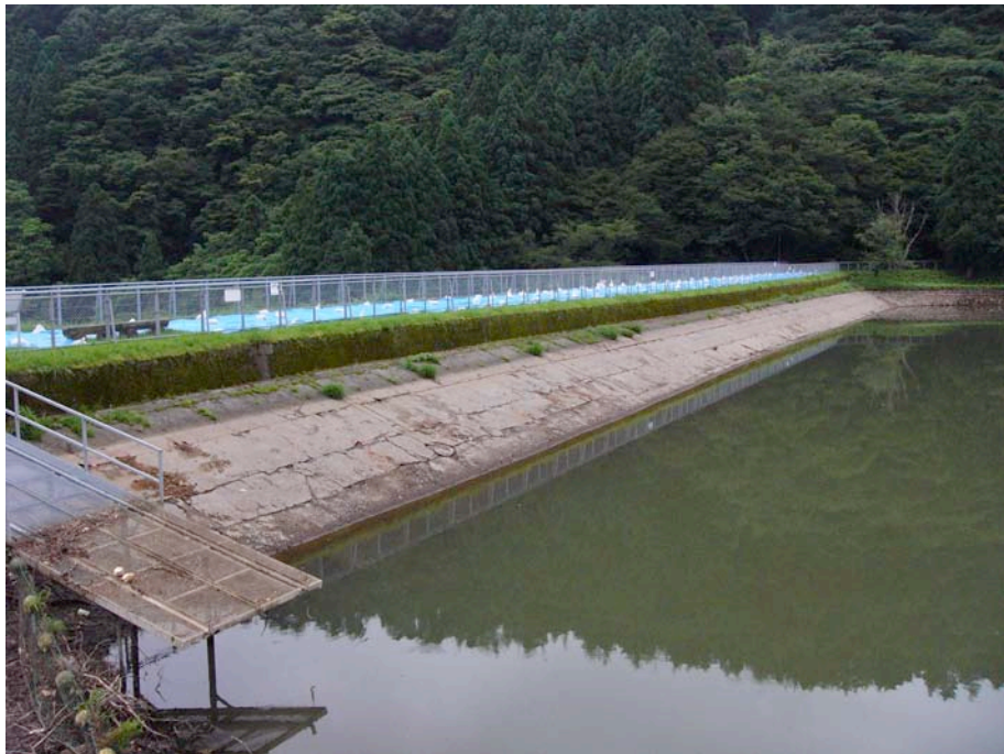
Figure 3.10: Embankment cracking at the crest of Kawauchi Dam, constructed in 1938. (Site YT19; N37.33635° E138.52410°, photos taken 7/21/07 at approximately 16:20).
