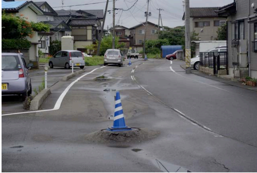
Figure 10.1: Example of an elevated manhole caused by settlement of road fill. The depression caused by densification of lightly compacted trench backfill during cyclic loading was evident along extensive sections of the roadway. This area was conspicuous for pipe breaks associated with ground deformation (Site SD11, N37.36650° E138.58868°, photo taken 7/23/07).
