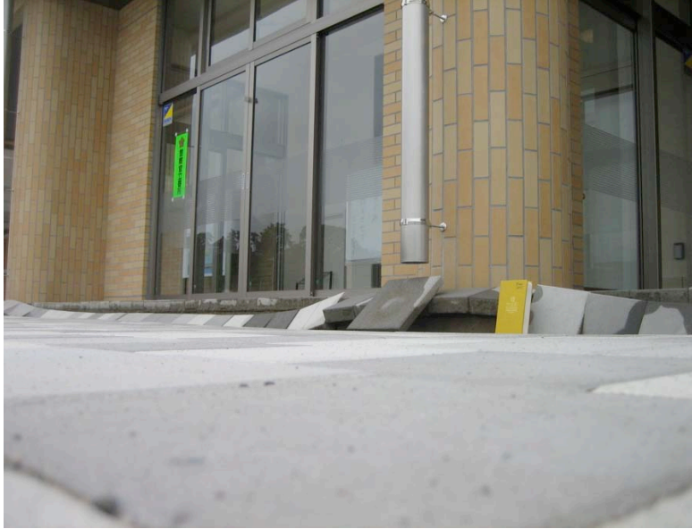
Figure 4.22: Kashiwazaki Harbor - The southern area experienced ground damage from liquefaction-induced lateral spreading and settlement. We observed settlement immediately adjacent to the pile supported port office building. (Site RK25, N37.36713° E138.53210°, 7/20/2007).
