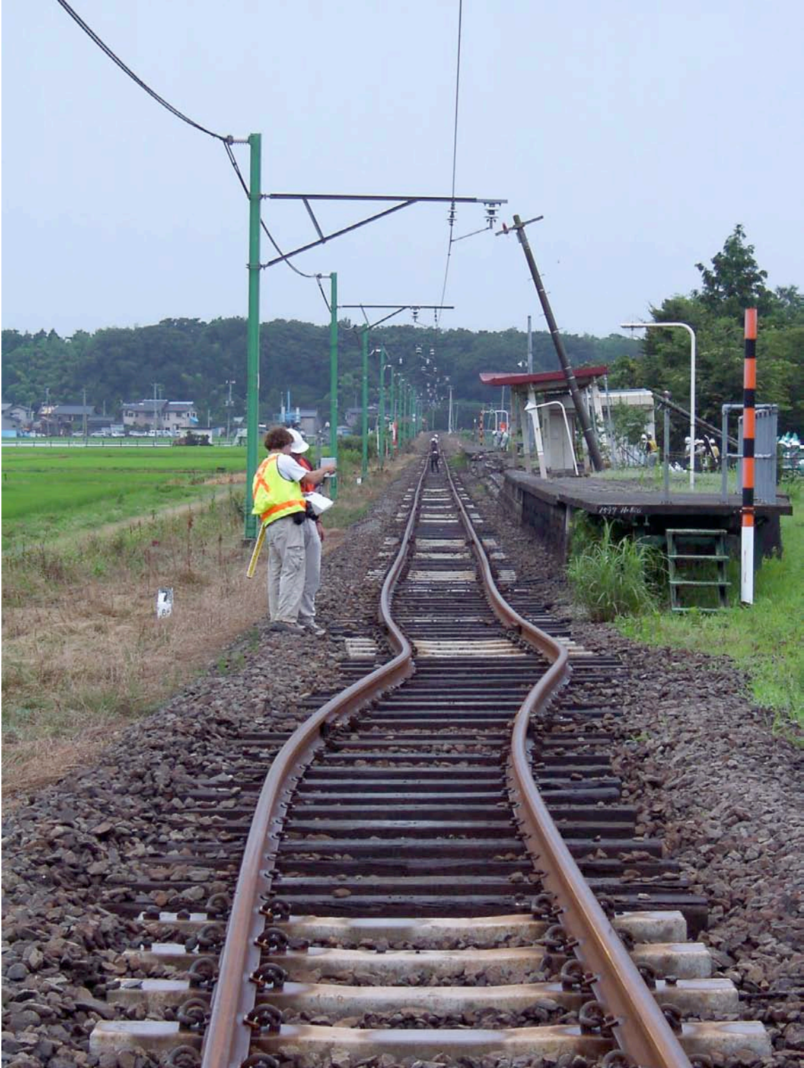
Figure 9.12: Lateral deformation of train tracks at Arahama Station (Site RK13, N37.40555° E138.60197°, 7/21/07 09:52).
