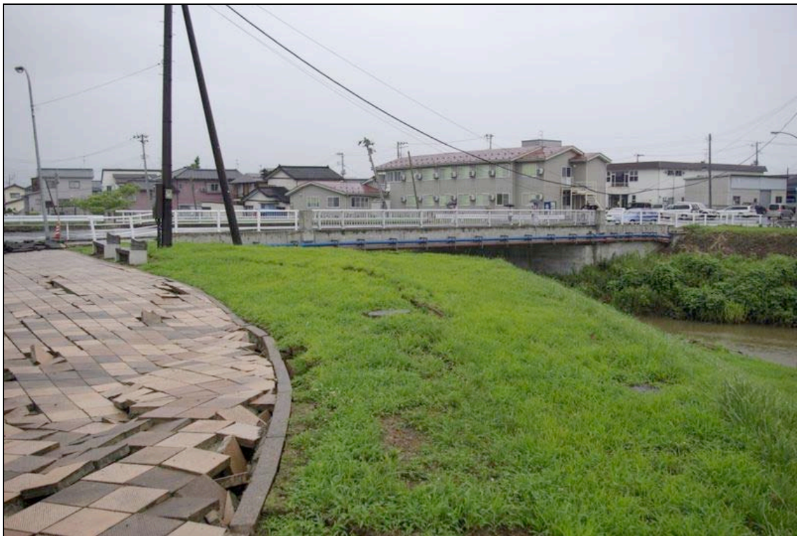
Fig. 6.32. Looking northwest at liquefaction of island and the Heisei Bridge.
