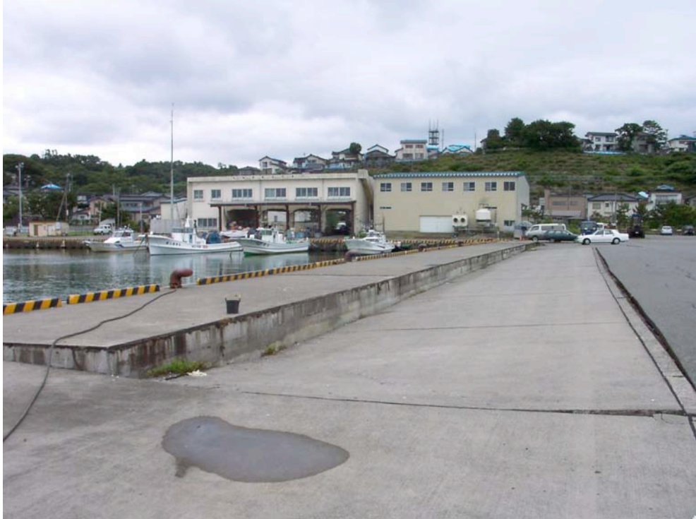
Figure 8.18: Kashiwazaki Port - East facing portion of the “Southwestern Pier” showing pronounced ground settlement (Site SD5, N37.36532° E138.53213°, photo taken 7/22/07 14:05).
