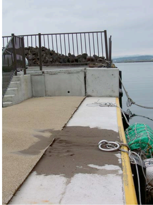
Figure 8.12: Kashiwazaki Port - Liquefaction-induced damage to the sightseeing wharf with minor displacement of the caisson quay wall (Site RK25/SA25/YT4, N37.36713° E138.53210°, photo taken 7/21/07 16:09).
