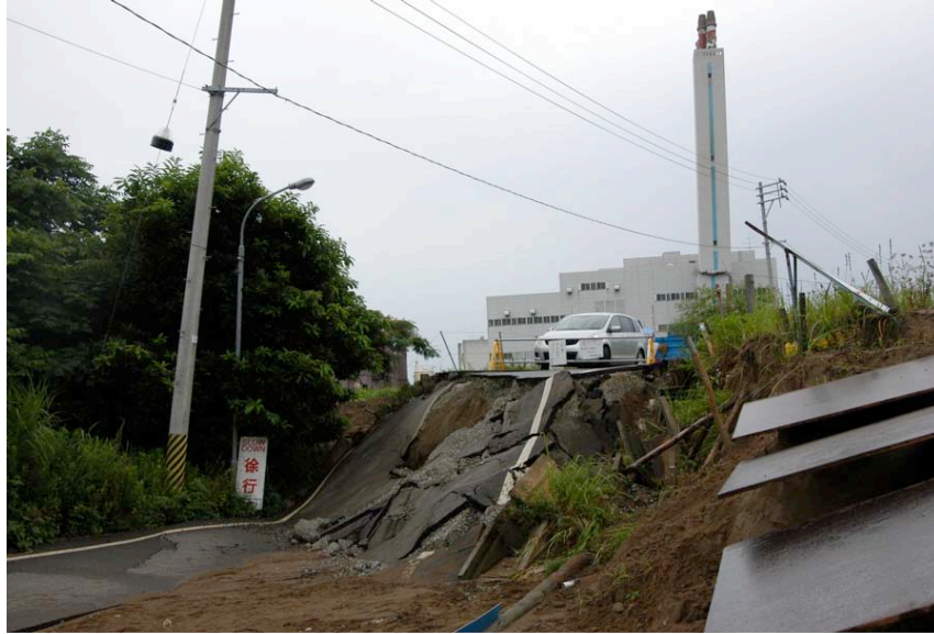
Figure 4.12: North side of Kai-Un Bridge area of the Sabaishi River - Lateral Spread on Road to Kashiwazaki Incinerator (Site RK6, N37.39343° E138.58555°, 7/19/2007). A zone of lateral spreading, sand boils and settlement crossing the present-day Sabaishi River, and that may be associated with a buried shoestring sand deposit of a former channel, resulted in failure of a road on the north side of the river adjacent to the Kashiwazaki Municipal Incinerator.
