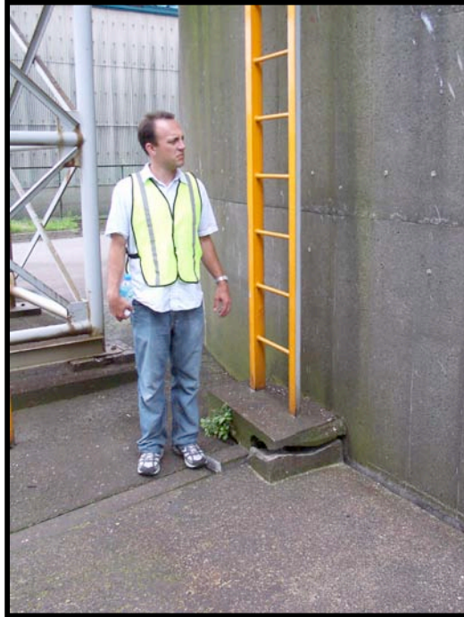
Figure 7.9: Kashiwazaki Port (Taiheiyo Cement Facility) - Evidence of minor to moderate settlement of sandy fill adjacent to one of the large diameter tanks (Site SD 9, approximately N37.36665° E138.53983°, photo taken 7/22/07 15:48).
