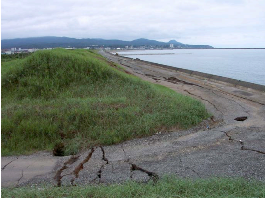
Figure 8.37: Ground deformations adjacent to the embankment and seawall (Location is southwest of Site SD1, photo taken 7/22/07 11:41).
