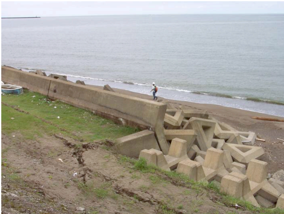
Figure 8.32: Eastern end of the seawall located adjacent to the damaged cement plant and mouth of the Sabaishi River (Site SD1, approximately N37.38868° E138.56413°, photo taken 7/22/07 10:56). Lateral spreading behind the wave armor units, as well as ground settlement and minor sea wall damage was widespread.
