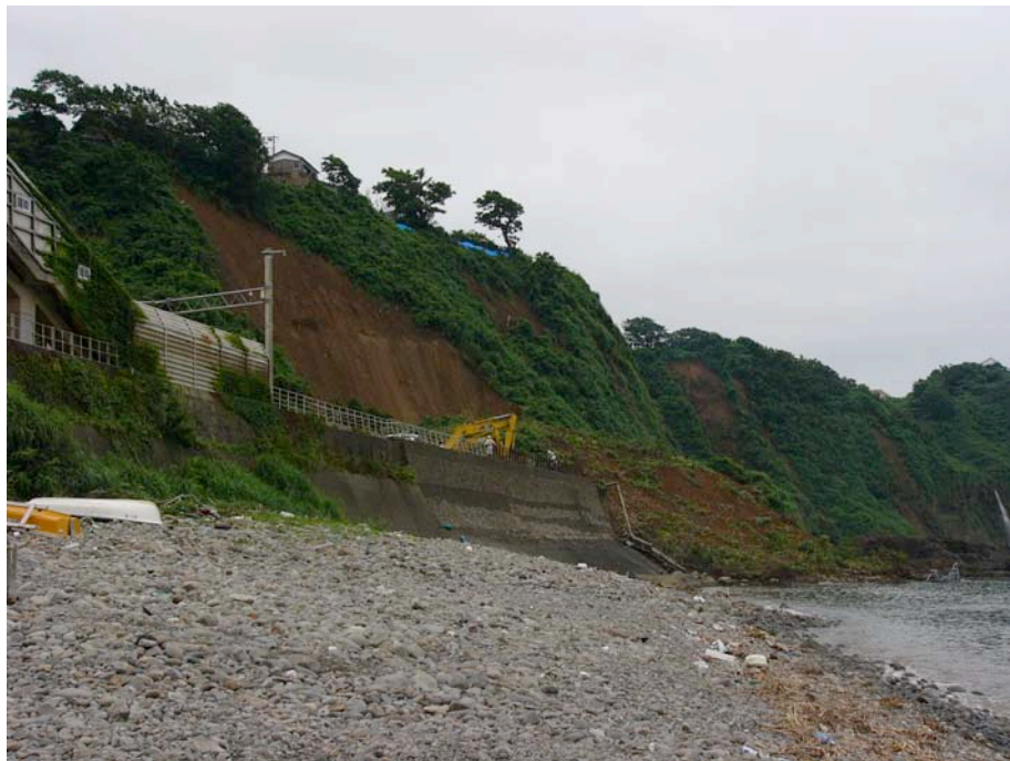
Figure 3.5: Landslide at the Oumigawa Train Station on the Shin-etsu Line (Site RK20/SA9/YT16; N37.34200° E138.48888°, photos taken 7/21/07 12:48 (top) and 7/24/07 15:00 (bottom)). This was among the largest of the coastal landslides to the south of Kashiwazaki. Site access was not possible due to construction repairs. Note that slope stability in this area has been a problem, as seen by the railway tunnel protection structure immediately behind (to the south) of this landslide. Many more smaller landslides were observed to the north and south of this location.
