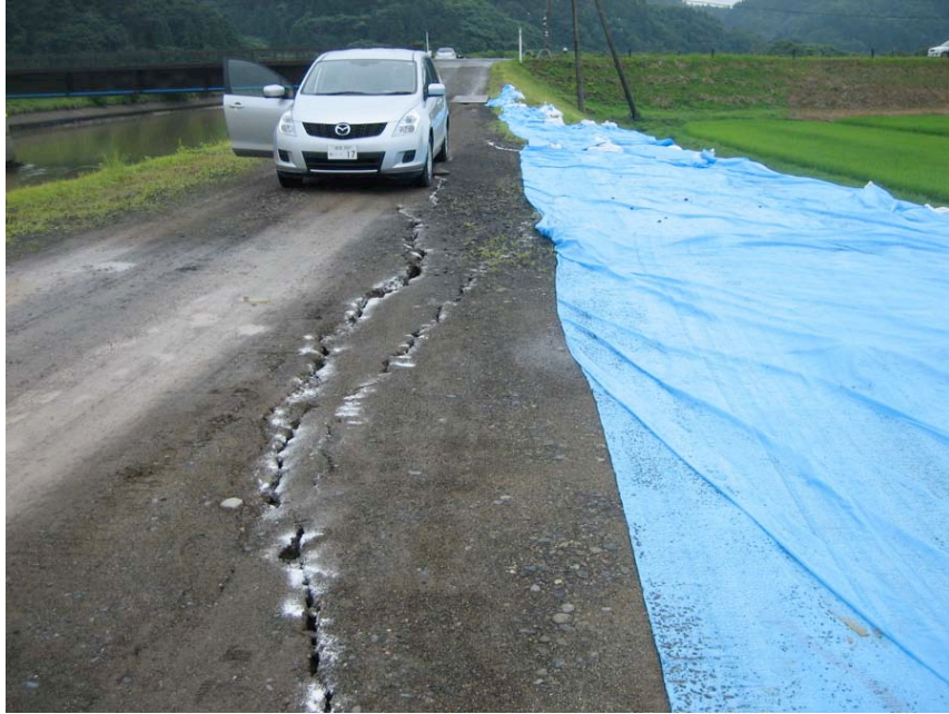
Figure 4.1: Fujii Weir downstream from Tashiou Bridge crossing of river. (Site RK16; N 37.34875^{\circ} E 138.61670^{\circ} , visited 7/21/2007 11:28 am UTZ+8). Extensive cracking of levee embankment.
