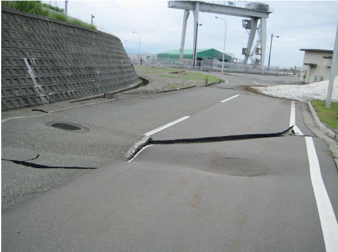
Figure 5.3: Damaged road at power plant.
