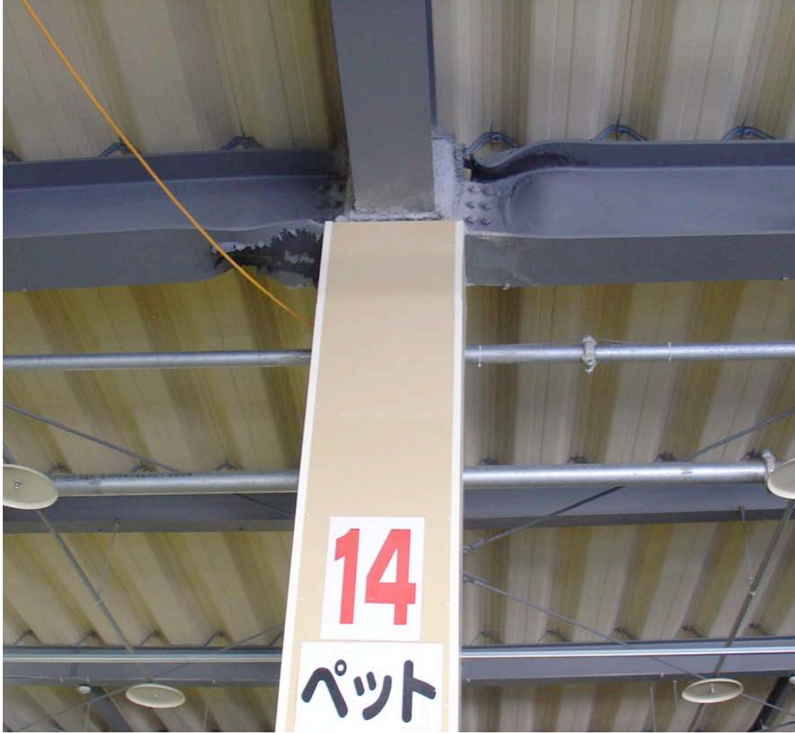
Figure 5.15: Buckling of beam flanges (Site RK41, N37.41472° E138.60833°, photo by Peter Yanev).
