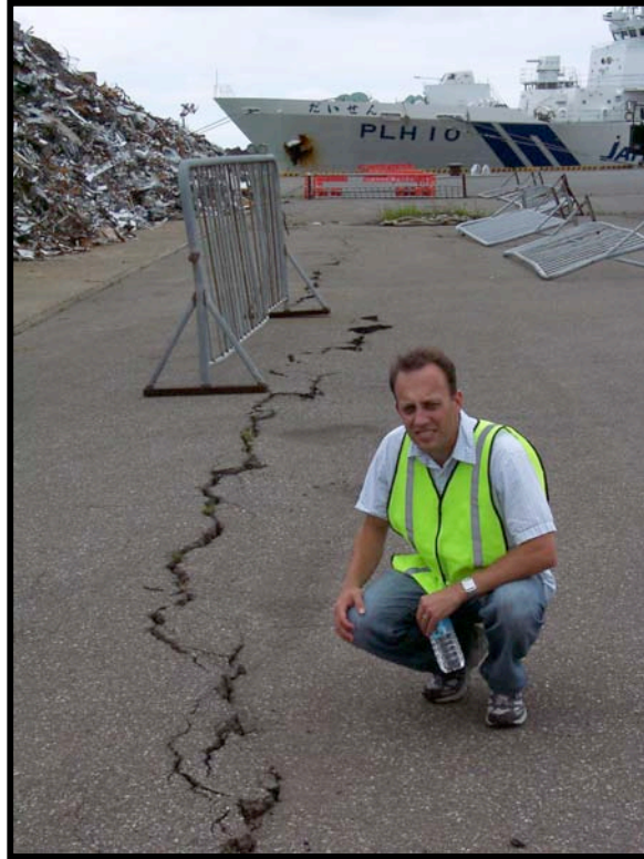
Figure 8.22: Kashiwazaki Port - Minor ground cracks located parallel to the western quay wall used as the berth for the Japan Coast Guard (Site SD8, N37.36680° E138.53825°, photo taken 7/22/07 15:17).
