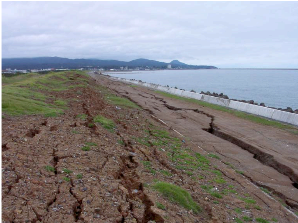
Figure 8.36: Representative cracking and lateral displacement of the clayey earth embankment adjacent to the seawall (Location is southwest of Site SD1, photo taken 7/22/07 11:35).
