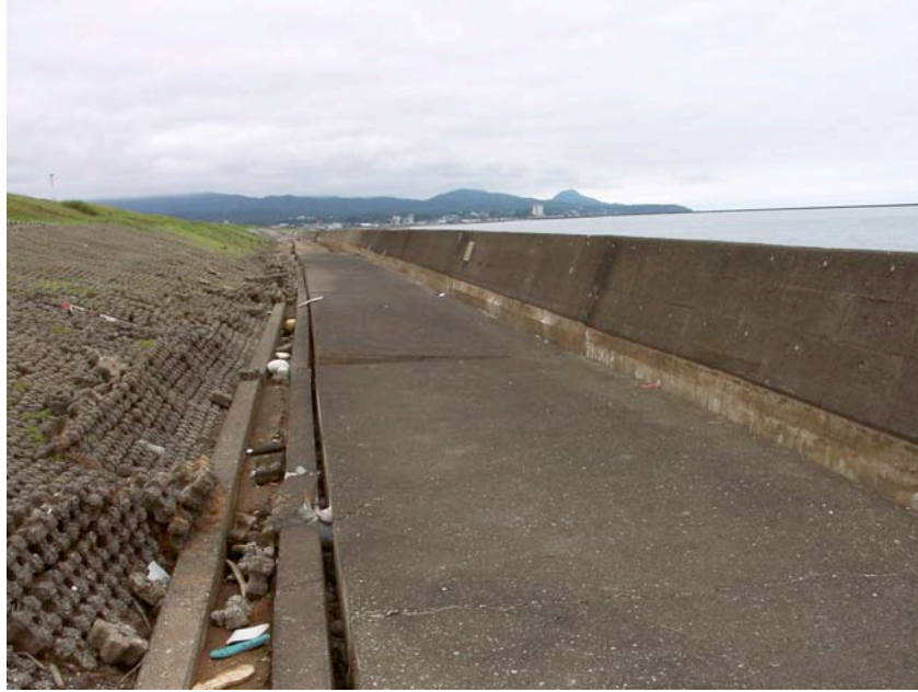
Figure 8.35: Evidence of seawall rotation, ground settlement, and longitudinal cracking of the benched embankment (Moving southwest of Site SD1, approximately N37.38868° E138.56413°, photo taken 7/22/07 11:25).
