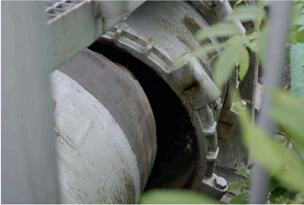
Figure 10.3: Damage to a water pipe at a stream crossing (Site RK4/YT3, N37.39233° E138.58063°, photo taken 7/20/07).
