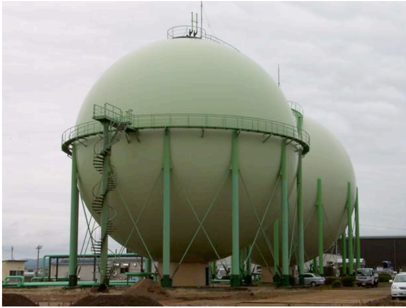
Figure 7.10: Steel natural gas tanks undergoing inspection by the operator and engineering consultants (Site SD13/RK57, N37.37253°, E138.59488°, photo taken 7/23/07 12:37). Trenching and below grade inspections had already taken place prior to the field investigation. No damage was observed to the tanks, pipe connections, or mains, however observations were made from the perimeter of the facility, a short distance from the structures.
