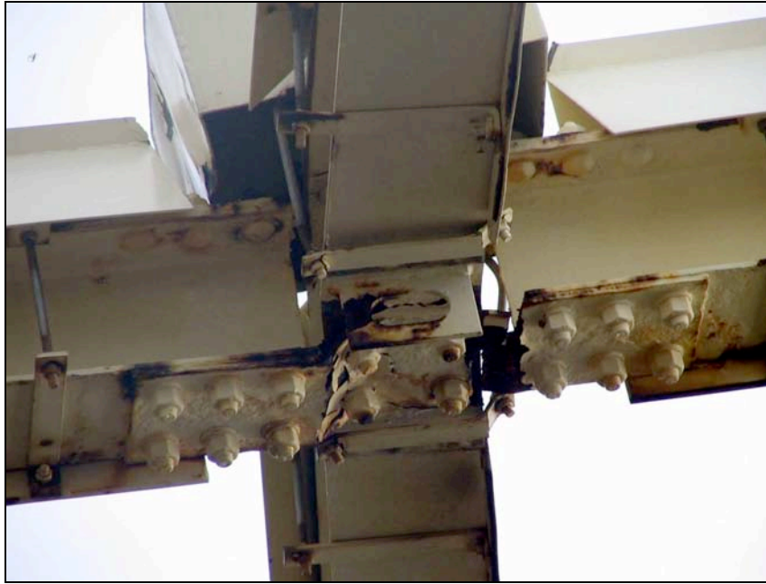
Fig. 6.26. Torn cross bracing connection on Yonahime Bridge.
