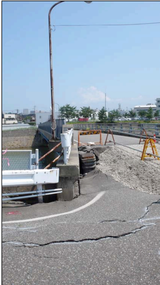
Fig. 6.62. Closer view of settlement at south abutment.
