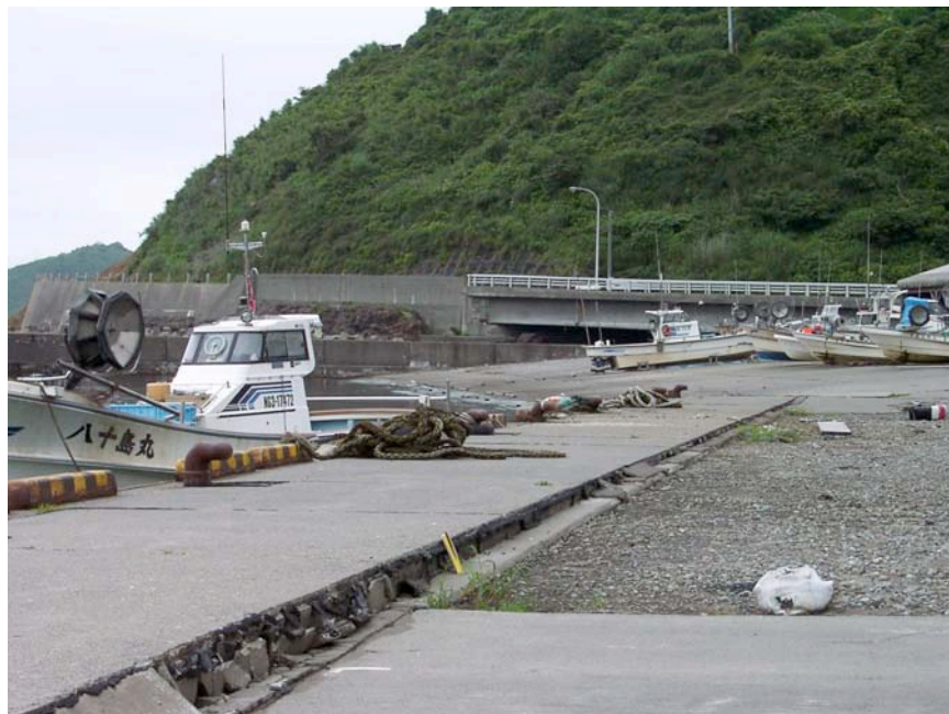
Figure 8.3: Kasashima Harbor - Settlement of fill behind quay walls (Site RK21, N37.33702° E138.46680°, photo taken 7/21/07 14:48).
