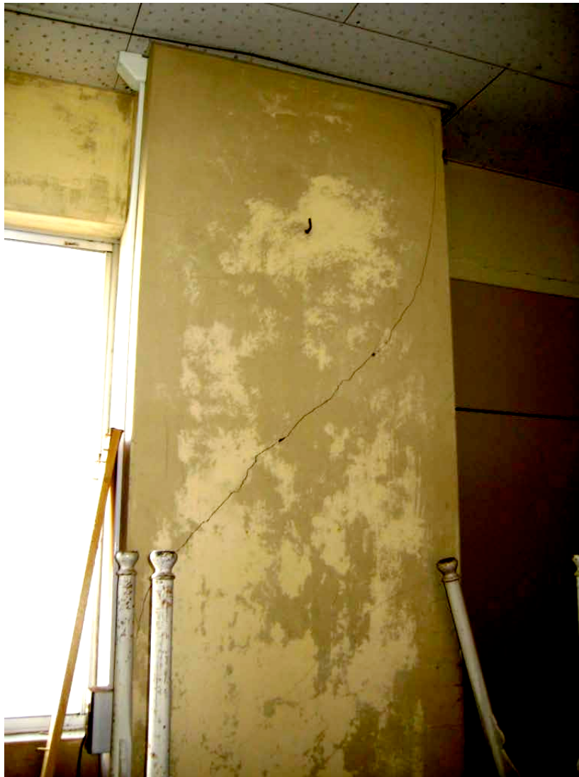
Figure 5.21: Column in first story of The Kashiwazaki High School, cross section and observed crack pattern (Site SP11, N37.3721°, E138.5569°).
