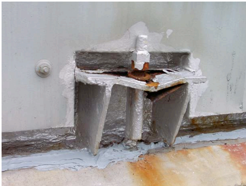
Figure 8.8: Kashiwazaki Port - Anchorage of asphalt storage tank (Located near Site RK25, N37.36713° E138.53210°, photo taken 7/22/07 12:37).
