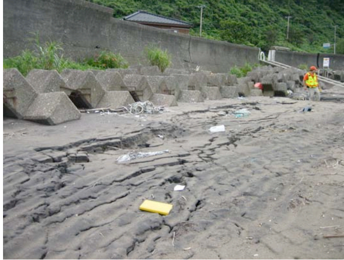
Figure 4.28: Liquefaction of beach sand resulted in lateral spreading, above, in front of a 30-meter-long segment of concrete seawall. (Site RK35, N37.48497° E138.626°, 7/22/2007)
