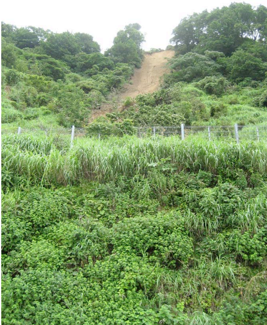
Figure 3.3: Coastal landslides on Highway 352 north of Kashiwazaki-Kariwa Nuclear Power Plant at road closure south of Route 373 (Site RK34-Slide 4; N37.48455° E138.62435°, photos taken 7/22/07 at approx. 10:45). This landslide is typical of many of those observed along the coast, and in this case did not damage transportation lines. Slide is approximately 10 m wide, 25 m long, and 0.5 m thick. Failure plane has approximate 50° inclination.
