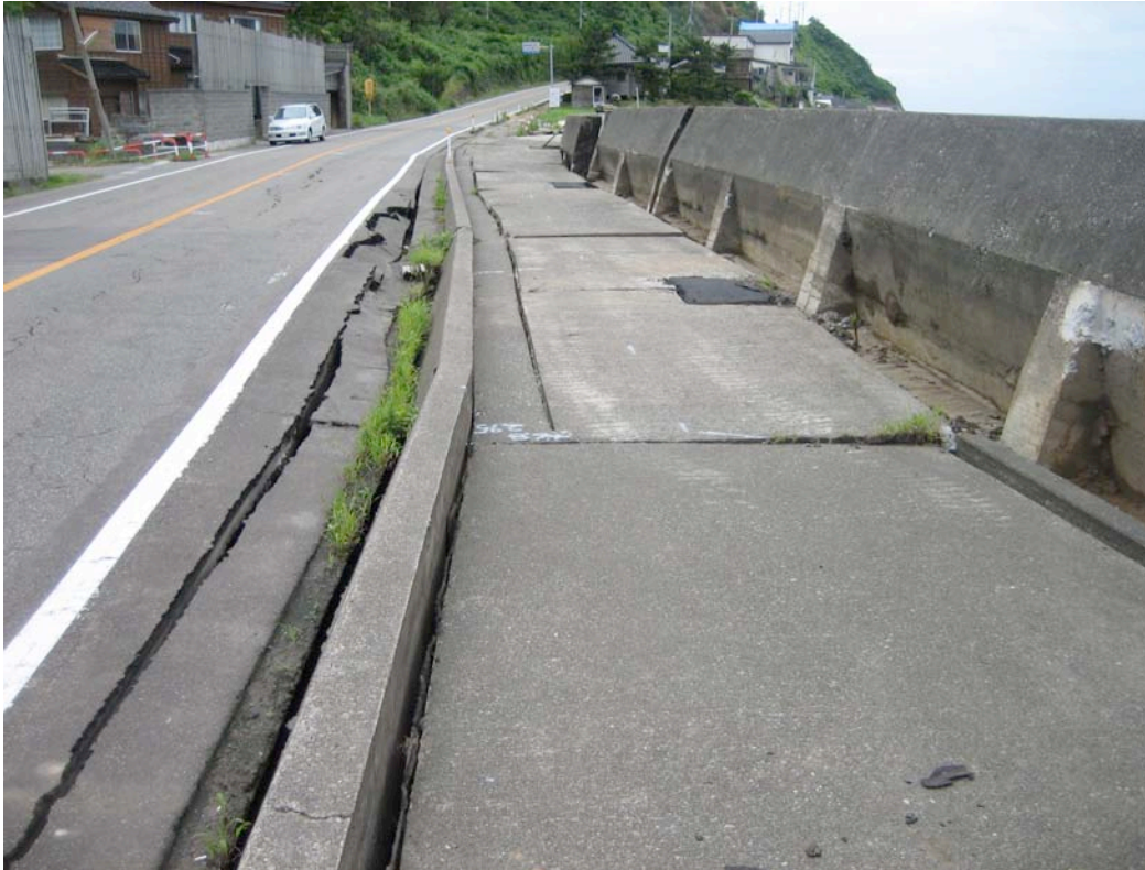
Figure 4.27: Liquefaction of beach sand led to lateral spreading of a road embankment and both rotation and translation of a 30-meter-long segment of concrete seawall. (Site RK35, N37.48497° E138.62645°, 7/22/2007).
