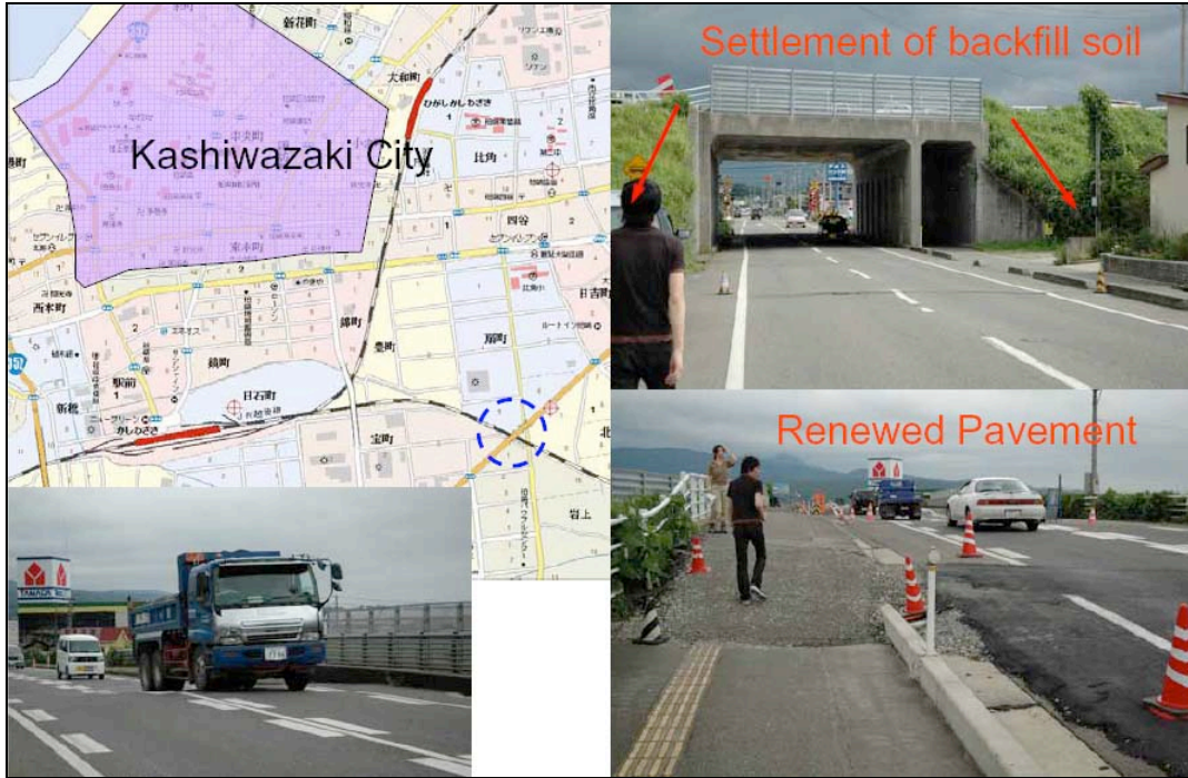
Fig. 6.16. Damage and repairs where Highway 8 crosses Route 522 Bridge (courtesy G. Watanabe, Tokyo Institute of Technology).
