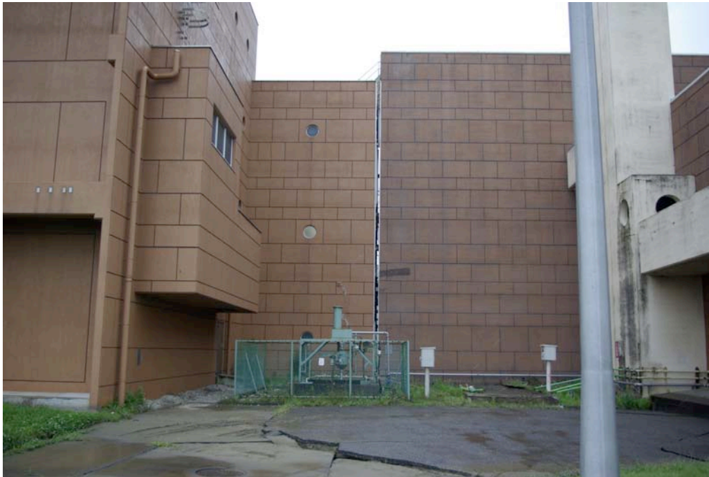
Figure 10.4: Ansui-Chou waste water treatment plant showing evidence of lateral spreading and extension of the structure (Site RK9, N37.38748° E138.56587°, photo taken 7/20/07).
