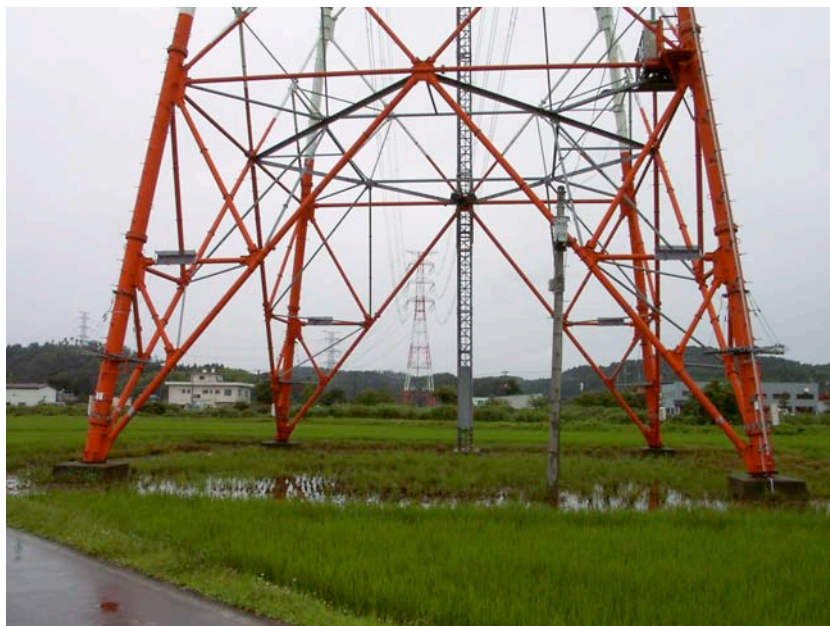
Figure 10.6: High voltage power line towers located in the Kashiwazaki area (Site RK12, N37.44113° E138.63390°, photo taken 7/21/07). No evidence of structural damage to the towers was observed.
