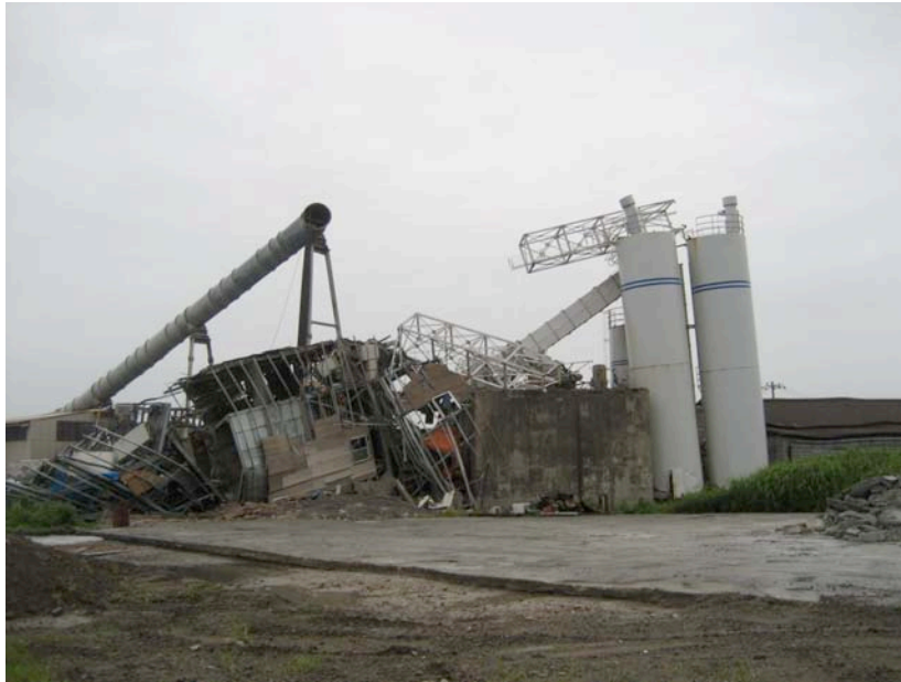
Figure 7.3: Damage to steel tanks at the cement plant located adjacent to the mouth of the Sabaishi River (Site RK10, N37.38795°, E138.56508°, photo taken 7/20/07 17:10). Tank damage likely caused by the cumulative effects of inertial loading, ground failures, and lateral loads due to the failure of appurtenant structures.
