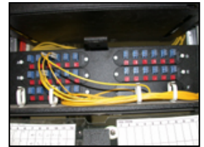
Pigtails provide various options with fiber optics and are a significant part of upgrades in North Las Vegas and at NTS.
