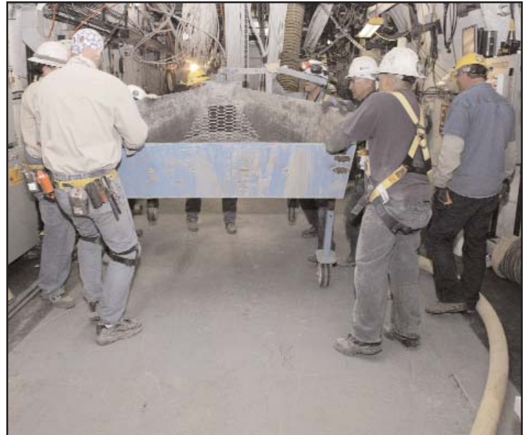
After the Krakatau subcritical experiment is lowered into the floor of the tunnel at the U1a Complex, marbles, gravel and cement seal the hole preventing radiation from the experiment escaping into the tunnel.
