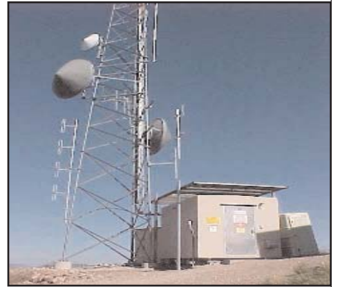
Lincoln County Microwave Communications Tower
