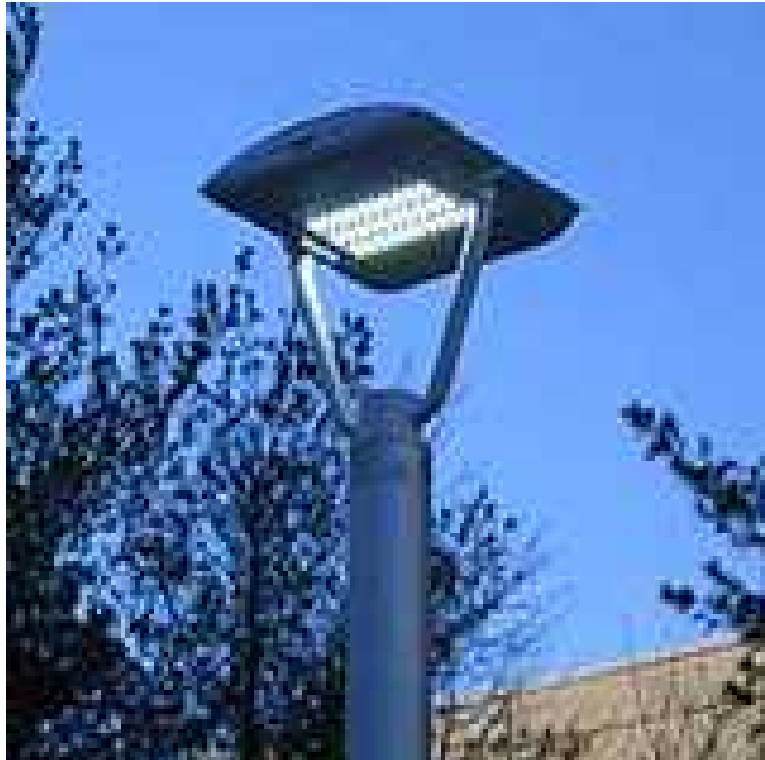
LED Walkway Lighting at the Federal Aviation Administration (FAA) William J. Hughes Technical Center in Atlantic City, New Jersey. http://www.netl.doe.gov/ssl/PDFs/Gateway_FAA.pdf
