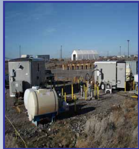
Polyphosphate Injection Pilot Test
