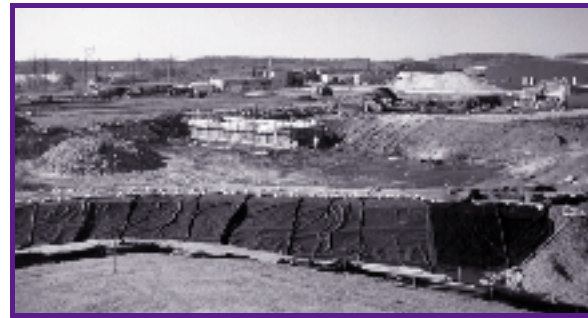
The Industri-Plex site in North Woburn, Massachusetts, illustrates Superfund’s effectiveness in returning sites to productive use. Once a contaminated property that threatened human health and the environment, the site is now poised to become a major commercial and retail district.
