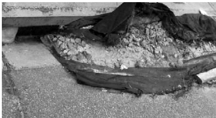
EPA is uncovering numerous storm water violations and is taking enforcement action to return violators to compliance (U.S. EPA photograph).
