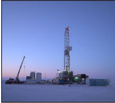
Final Construction Phase of Drill Site Camp, December 2002 (Photo by Hideaki Takahashi, Japex Canada Ltd. Reproduced with the permission of the Minister of Public Works and Government Services Canada, 2002 and courtesy of Natural Resources Canada, Geological Survey of Canada. )
