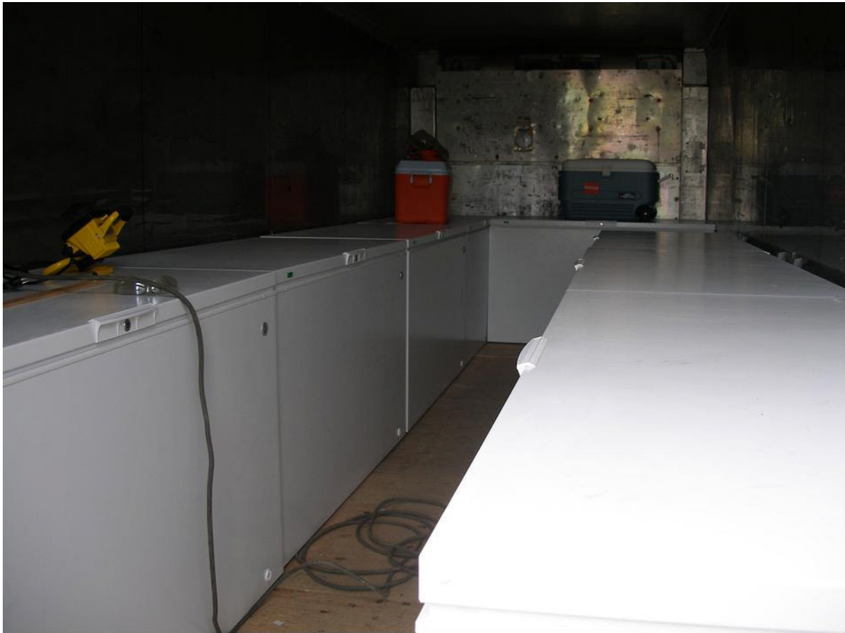
Figure 3: 6 of 8 Freezers installed for core storage in refrigerated unit prior to temporary disconnection of unit for installation of man-door, electrical outlets, and lighting (May 16, 2007).
