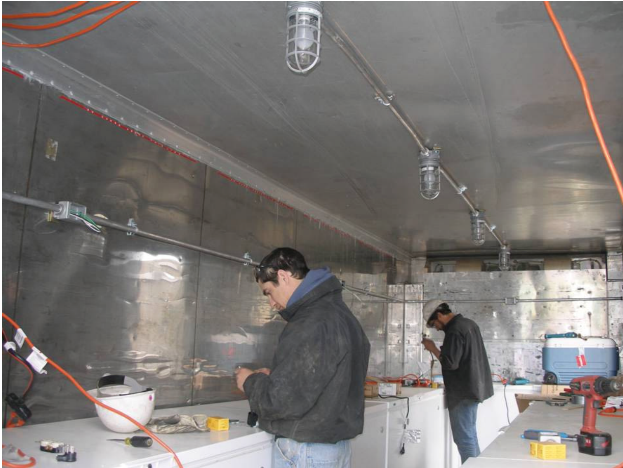
Figure 4: ASRC electrical and construction staff modifying core storage refrigerated unit for lighting, electrical outlet, and man-door. Extension cords visible in photo were for temporary power to freezers to keep core cold during unit modification (May 16, 2007).
