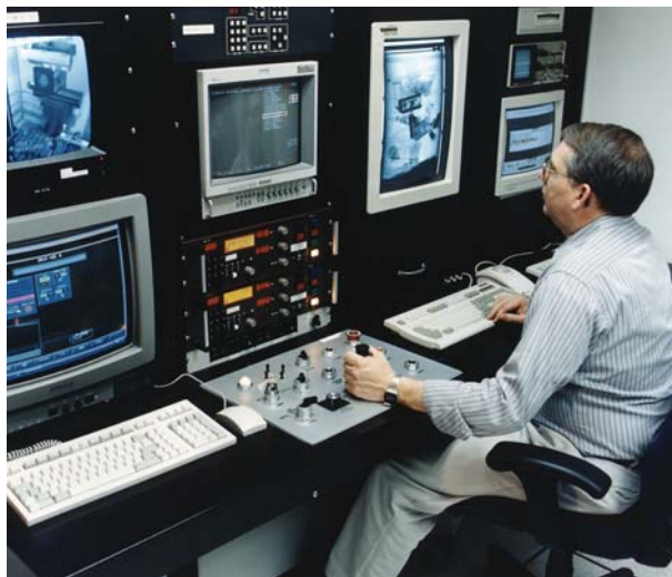
Control console at the Waste Receiving and Processing Facility at Hanford. Hanford's solid waste processing facility is the first in the Department's nation-wide complex built to handle transuranic wastes. The waste containers are staged, inspected by x-ray, and contents are assayed to determine the quantity of radioactive materials present.
