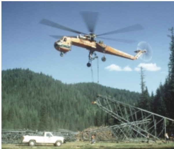
Construction of Taft-bell towers. The Bonneville Power Administration is the Federal agency created by Congress in 1937 to sell and deliver power from the Bonneville and Grand Coulee dams.
