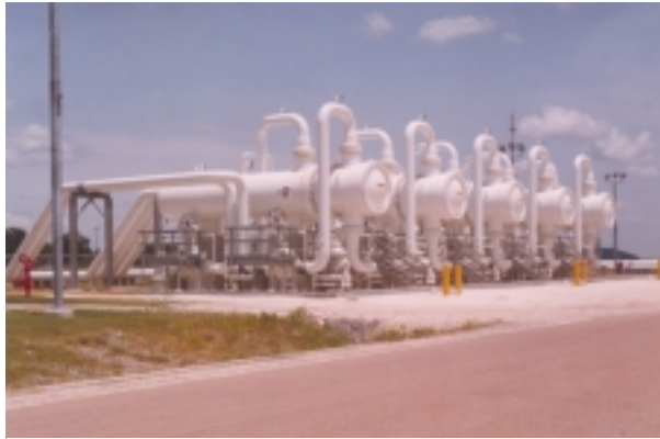
Strategic Petroleum Reserve West Hackberry Heat Exchangers.
