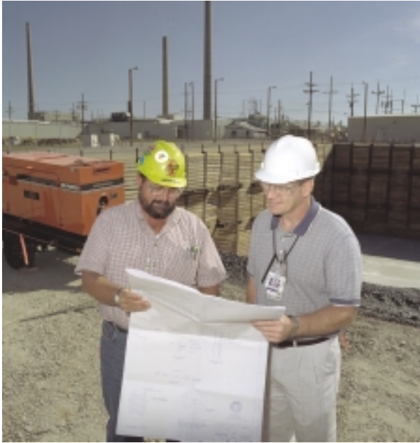
Excavation began during 2000 for the National Nuclear Security Administration's Tritium Extraction Facility at the Savannah River Site. The facility is being constructed to safely and efficiently extract tritium, a radioactive form of hydrogen gas, from rods that have been irradiated for 18 months beginning in Fiscal Year 2004 in Tennessee Valley Authority reactors. Tritium is a vital, but perishable component of the United States' nuclear weapons.
