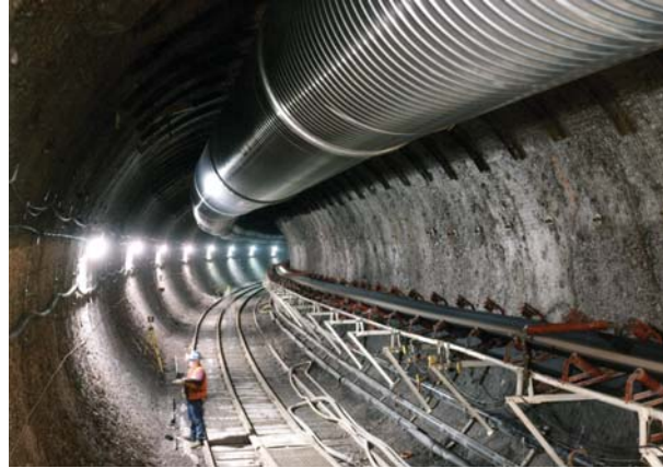
View of an exploratory tunnel dug by the 25-foot-diameter tunnel boring machine at Yucca Mountain.
