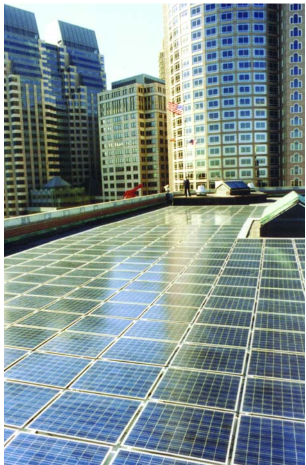
Photovoltaic system, consisting of 372 solar panels on the roof of the Williams Building, Boston, Massachusetts.
