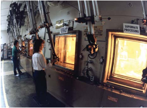
Savannah River Site technicians working at high-level waste cells. Work at the high-level cells includes miscellaneous testing, proving, sampling, and analysis of radioactive materials originating at Savannah River and other Departmental facilities.
