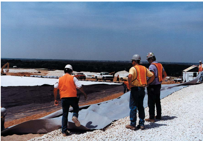
Safety officials monitor the installation of the high density polyethylene (HDPE) liner on the disposal cell as part of the good safety practices at the Weldon Spring Site.
