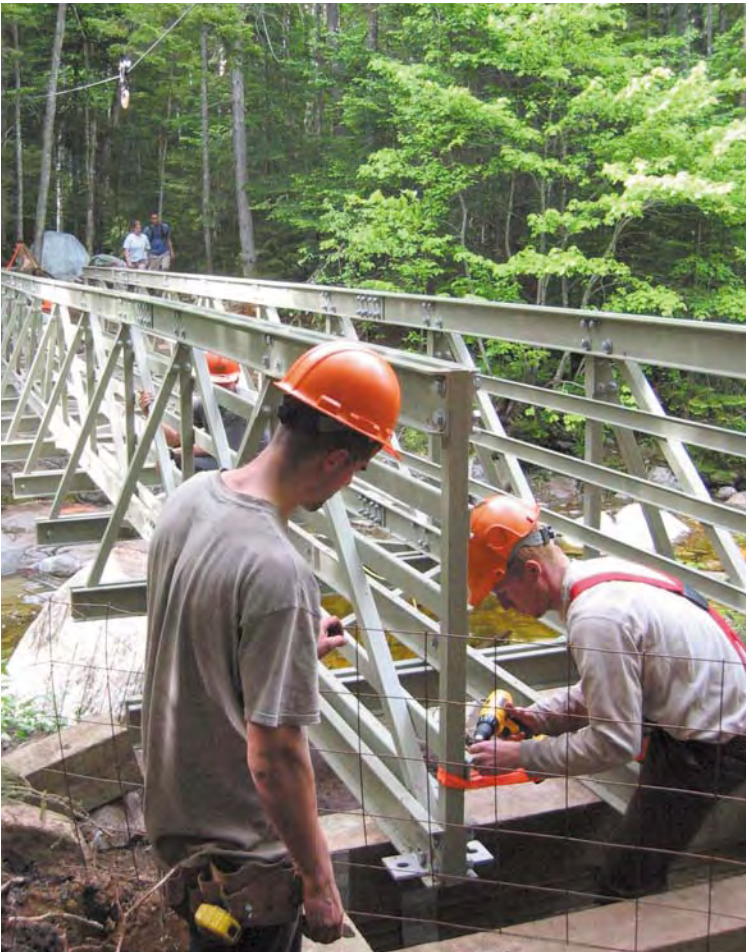
With support from the Appalachian Trail Conservancy and NPS, a new bridge is installed over Cascade Brook in New Hampshire by an AMC trail crew – Appalachian Mountain Club
