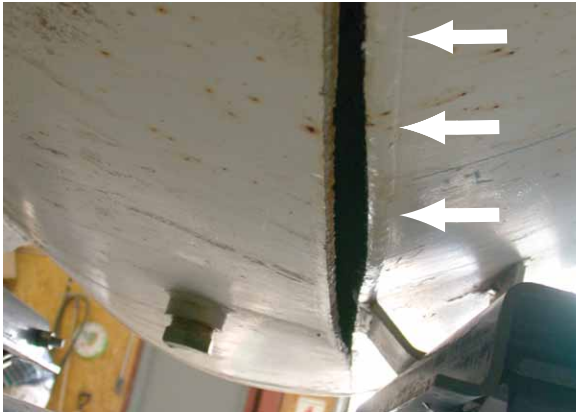
Figure 4. Fracture running beside, to the left of, longitudinal weld (line of weld is marked with arrows).
