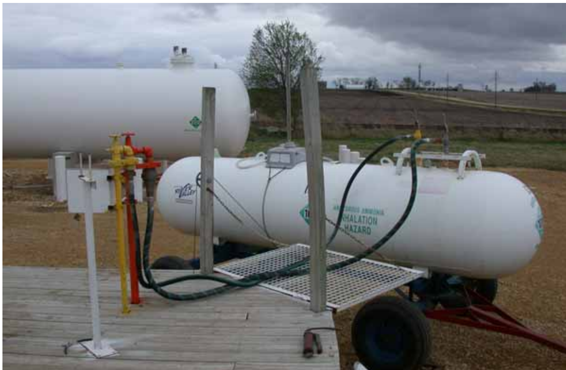
Figure 7. A nurse tank hooked to loading hoses.
