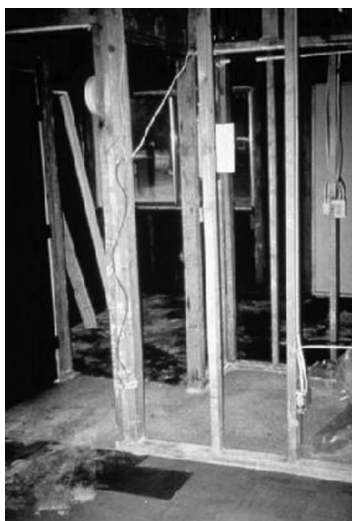
Figure 5. Residences with drywall removed.
