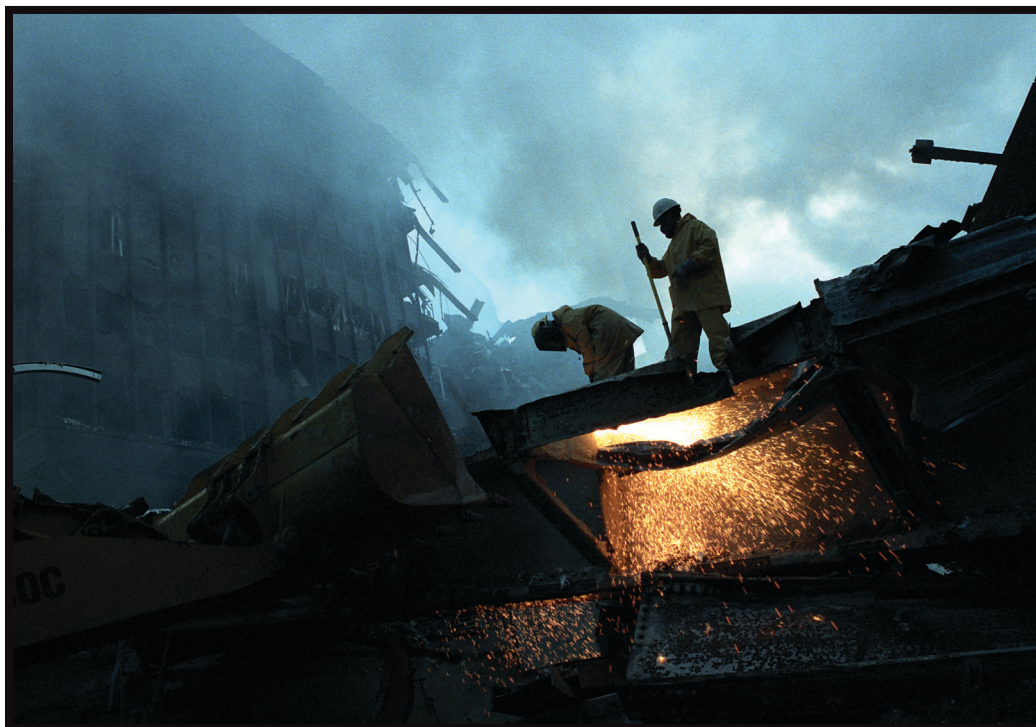
Dangerous days. Ironworkers balance precariously as they cut through the rubble of the World Trade Center.
