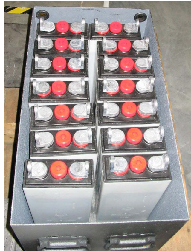
Lead-Acid Battery Cells from an Avista PEM fuel cell
