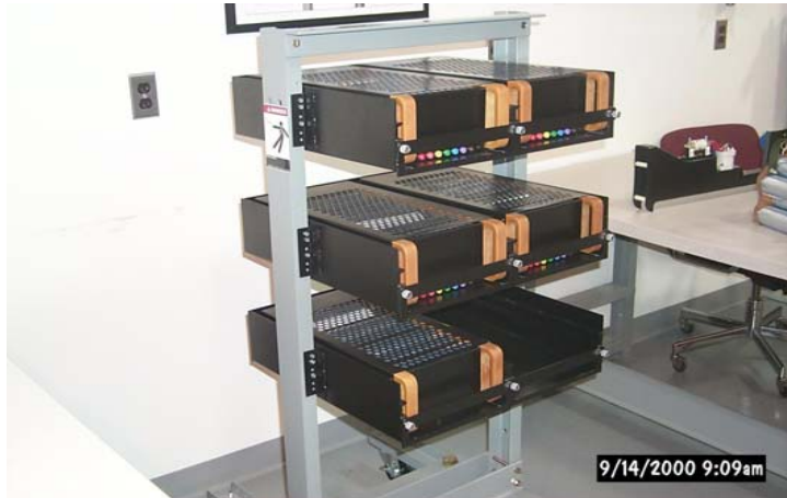
Lithium Battery modules
