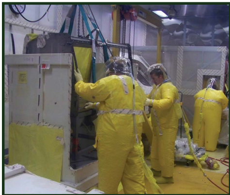
Workers in protective equipment remove a glovebox section after cutting open an oversized box.
