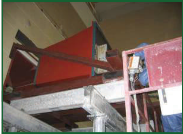
A specially designed and fabricated extraction tool was used to remove the lead glass windows from the wall.
