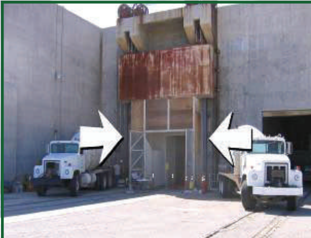
Steel columns now stabilize the two sections of the blast door in the open position .
