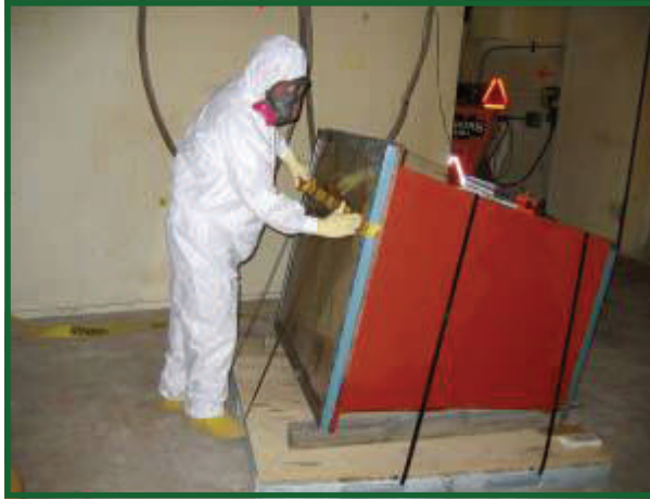
Strict procedures and diligent work allowed the task to be performed with zero safety incidents.
