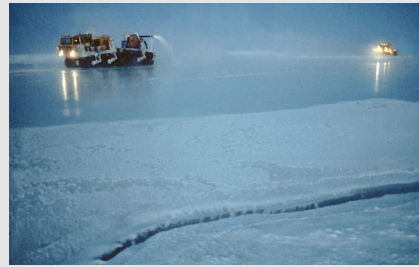
Big footprints. An ice road being constructed in the North Slope region is an example of the types of industrial "footprints" created by oil extraction that concern environmentalists and others.
