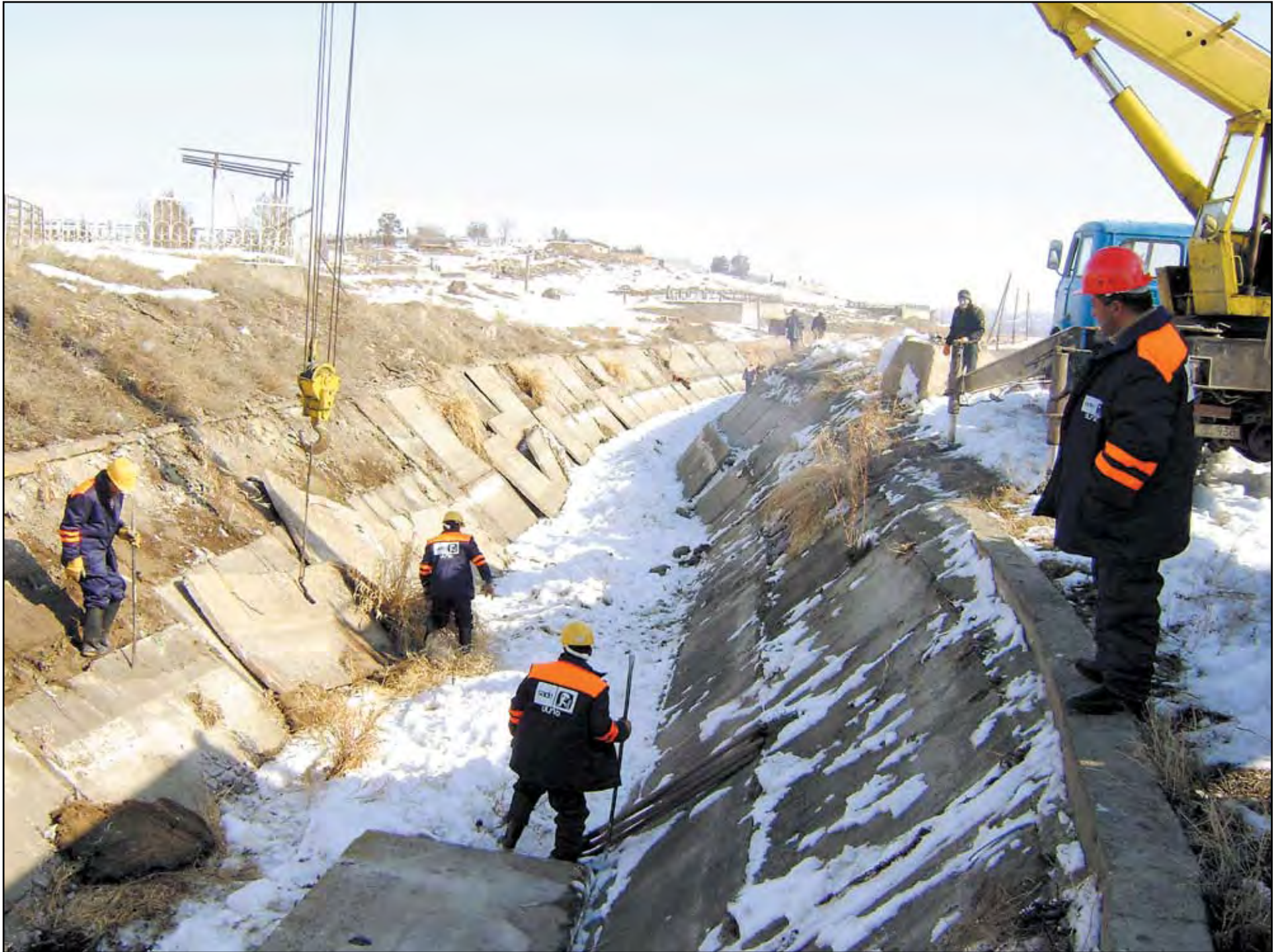
Construction on the Arzni-Shamiram waterway, Jan. 29, 2009. Photo: Armen Hakobyan for the Armenian Reporter.
