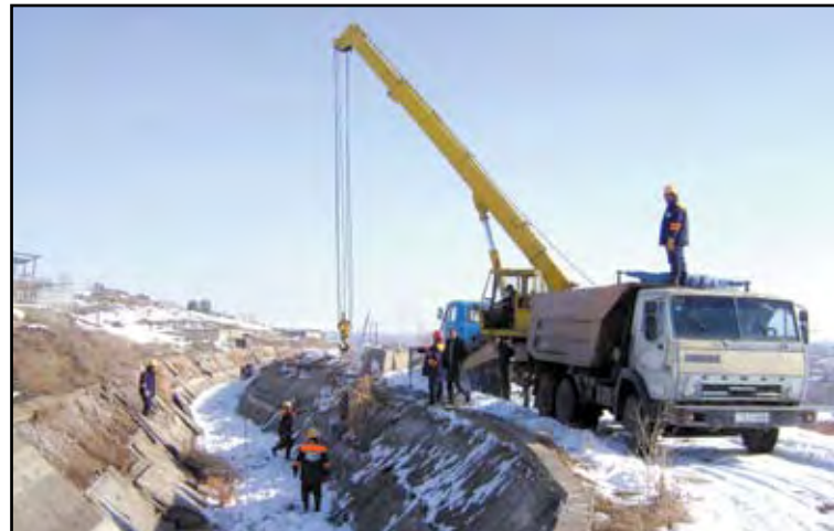
A construction crew renovates the badly damaged Arzni-Shamiram canal. Photo: Armen Hakobyan for the Armenian Reporter.
