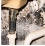
Mold on drywall under leaky sink. (photo, John Martyny, Ph.D.)
