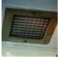
Example of exhaust vent in a bathroom. (photo, Terry Brennan)
