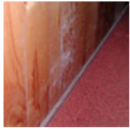
Mold on wooden paneling. (photo, Terry Brennan)
