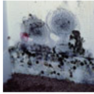
Moldy bedroom closet. Water condensed from the air onto the gypsum board. The wall is cool enough for condensation because there is a hole in the insulation and it is cold outdoors. (photo, Terry Brennan)
