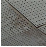
Acoustic ceiling tiles with water damage. (photo, Terry Brennan)
