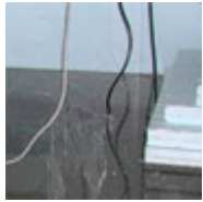
Several inches of water in a basement with a broken sump pump. (photo, Terry Brennan)
