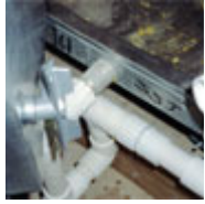
Example of a drain pan beneath a cooling coil that slopes to a drain line and is constructed of stainless steel. (photo, Terry Brennan)
