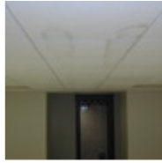
Water-damaged ceiling tiles. Air conditioning ducts above the ceiling were not insulated in several areas resulting in condensation on the ducts that dripped onto the ceiling tiles. (photo, Terry Brennan)
