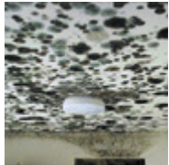
Extensive mold contamination of ceiling and walls. (photo, Terry Brennan)
