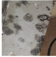
Sections of moldy gypsum board. (photo, Terry Brennan)
