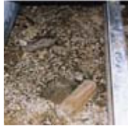
Mineral deposits on the surface of a dirt crawl space caused by chronic water problems. (This is not mold.) (photo, John Martyny, Ph.D.)
