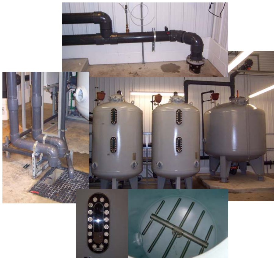
Figure 4-3. Treatment System Components
