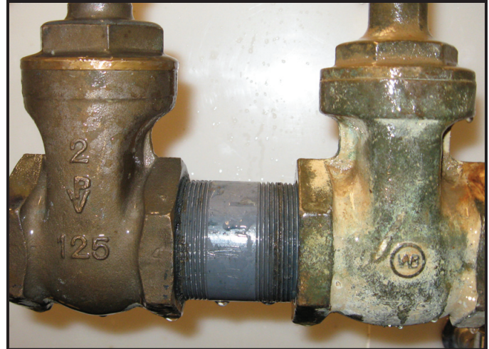
Unaccounted-for water includes conveyance losses and public uses.
