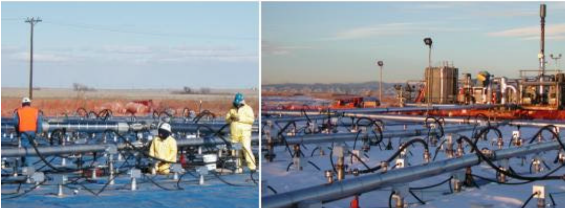
Figure 5 – Photographs of Installation and Operation of Hex Pit ISTD Well Field. Several inches of snow cover the surface seal. In the foreground of photo at left is a row of heater-only wells (shorter wells with electrical junction boxes on top). In the left foreground of photo at right is a heater-vacuum well (taller well with black vapor extraction line leading into jacketed and insulated horizontal manifold piping). The AQC system in the background of the photo at right includes thermal oxidizer in rear center (behind light stand); blowers and stack are at right.
