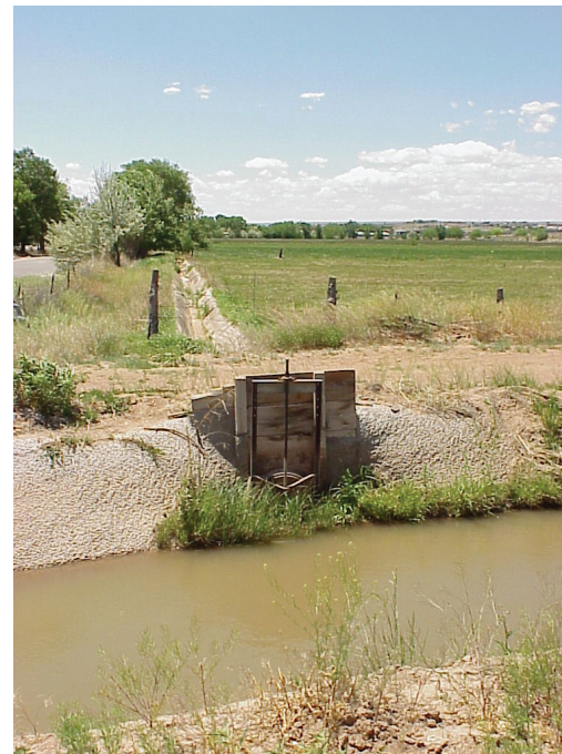
The headgate of an acequia (or ditch) near Paseo del Norte in northern Albuquerque.
