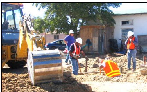
LUST Site Assessment on the Hopi Indian Reservation conducted through the national LUST cleanup contract
