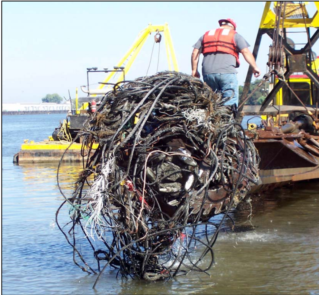
Figure 10. Debris fouling of cutterhead by cables.
