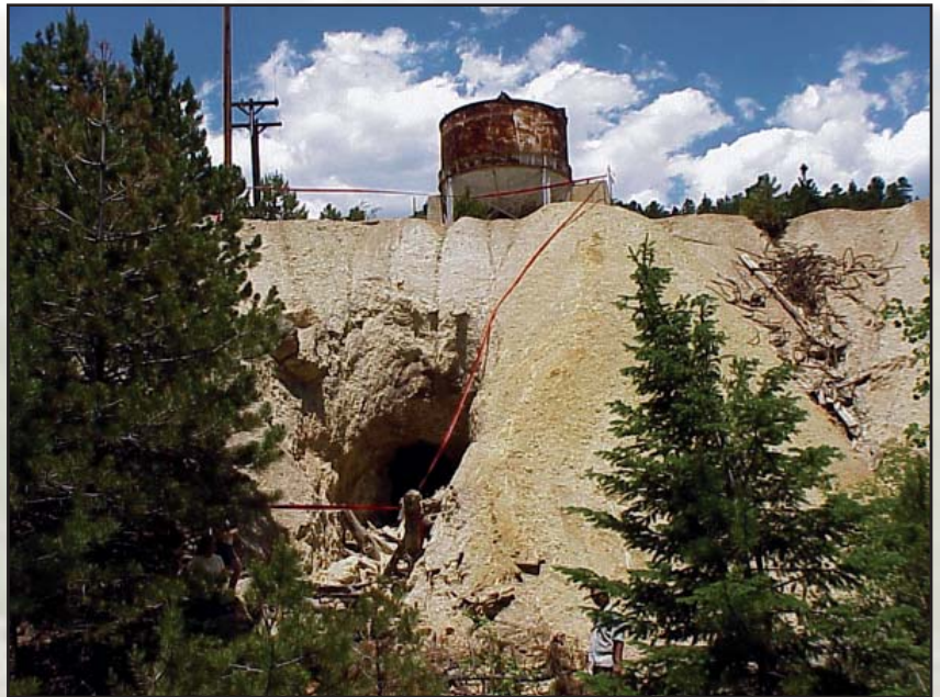
Open mine pits and deteriorating structures create safety hazards
