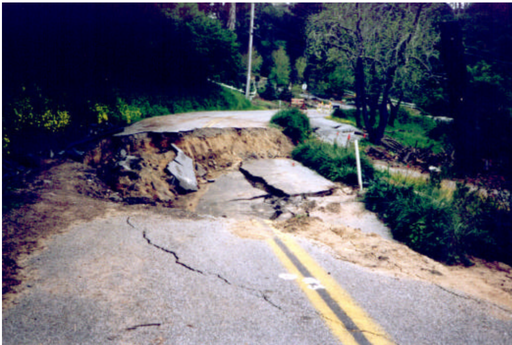
Figure 2b. Example of photographic record. Typical roadway damage in Santa Cruz County. (Photograph courtesy of R. Baum, USGS.)
