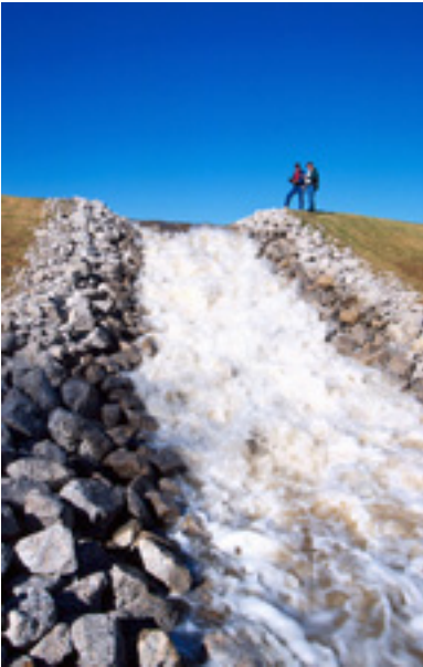
This rock chute safely transfers runoff to a lower elevation.
