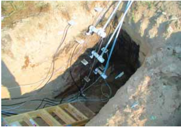
Figure 4. Instrumentation installed in the unsaturated zone at a site near Bemidji, Minnesota, to estimate recharge using the UZWB method.
