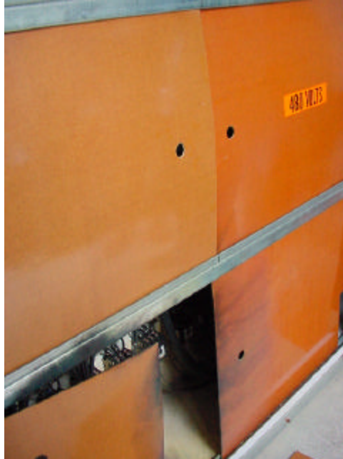
Exhibit 2. Dislodged Micarta Insulating Panel
