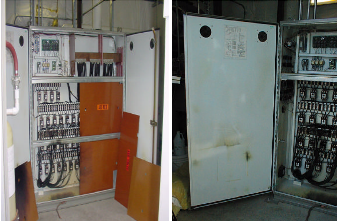
Exhibit 7. Sliding Panels, Vent, and Fan
