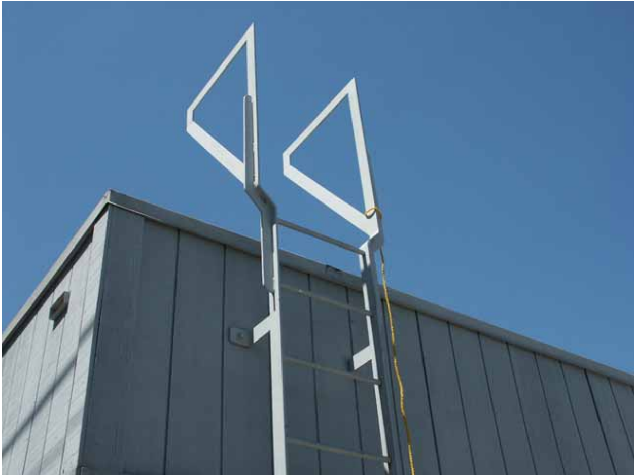
Figure 3.1.5-1: The walkthrough section of the ladder showing the angle-iron configuration of the side rails.
