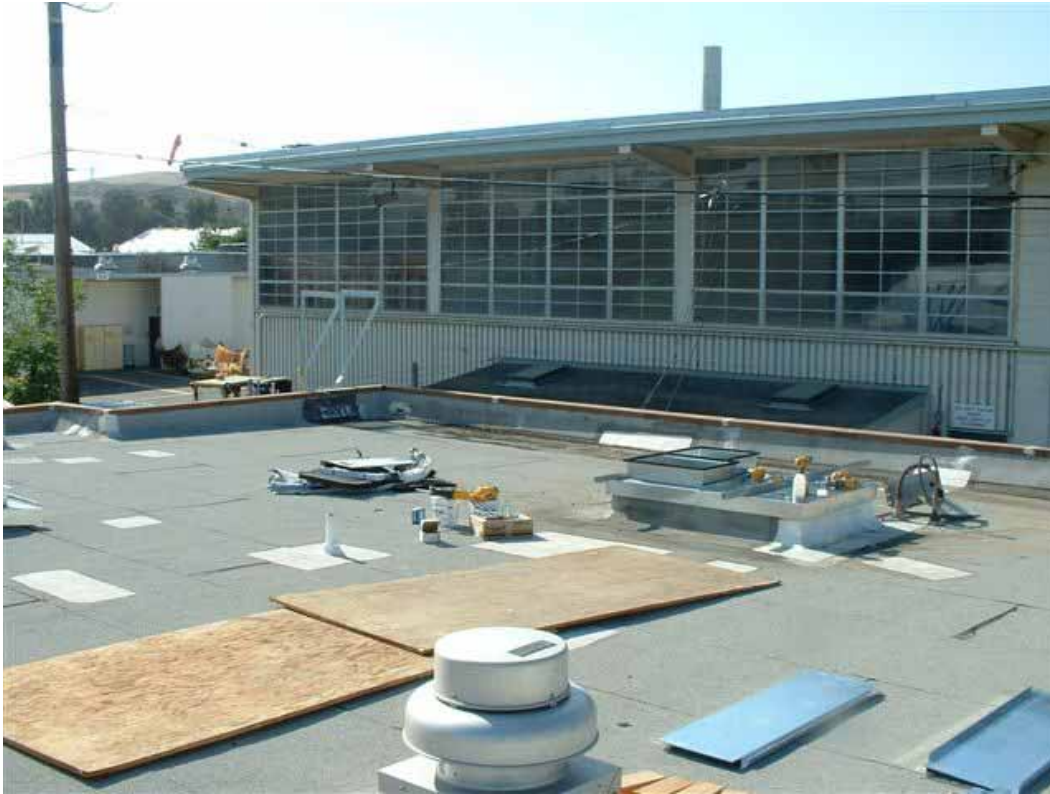
Figure 1.2-2: The roof of the building where the accident occurred, showing the ladder walk-through to the roof and general work area. The location of one of the air conditioning units is visible, although the unit was removed at the time the photograph was taken.
