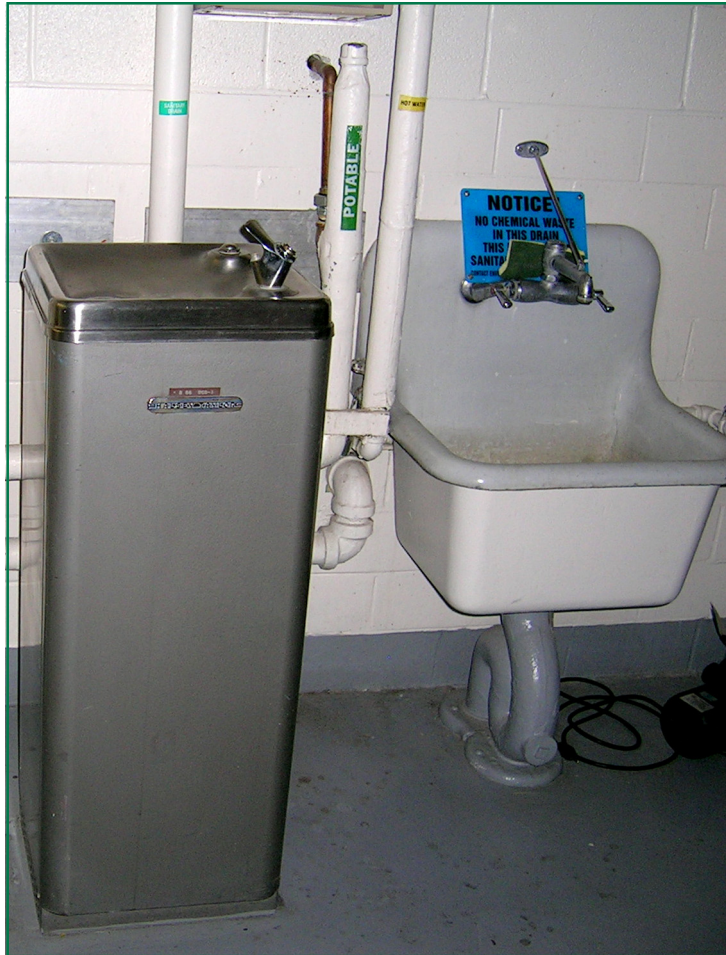
Exhibit 2.9-3 The utility sink found to be contaminated in R3. The drinking fountain was not contaminated.
